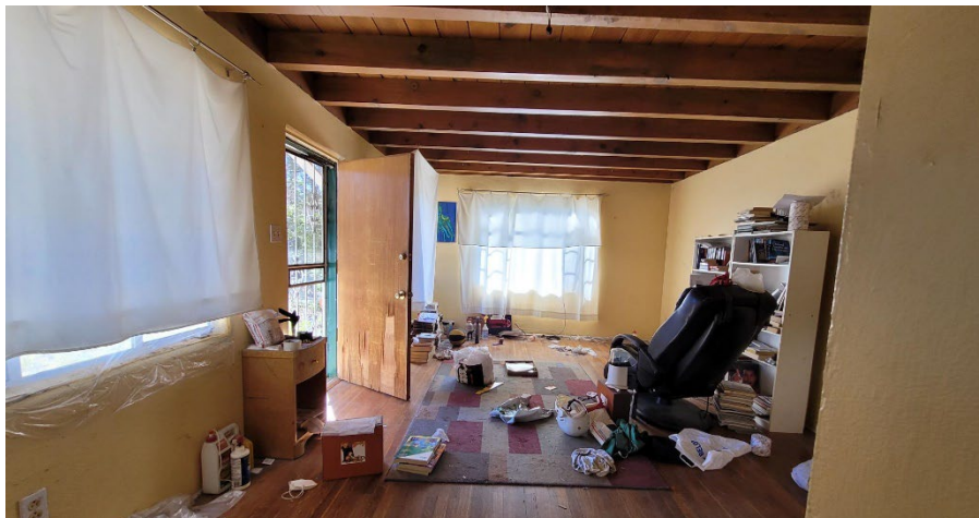
Top left: exposed wiring at the exterior of the main house; top right: structural cracks in the main house; bottom: one of the rental units.
