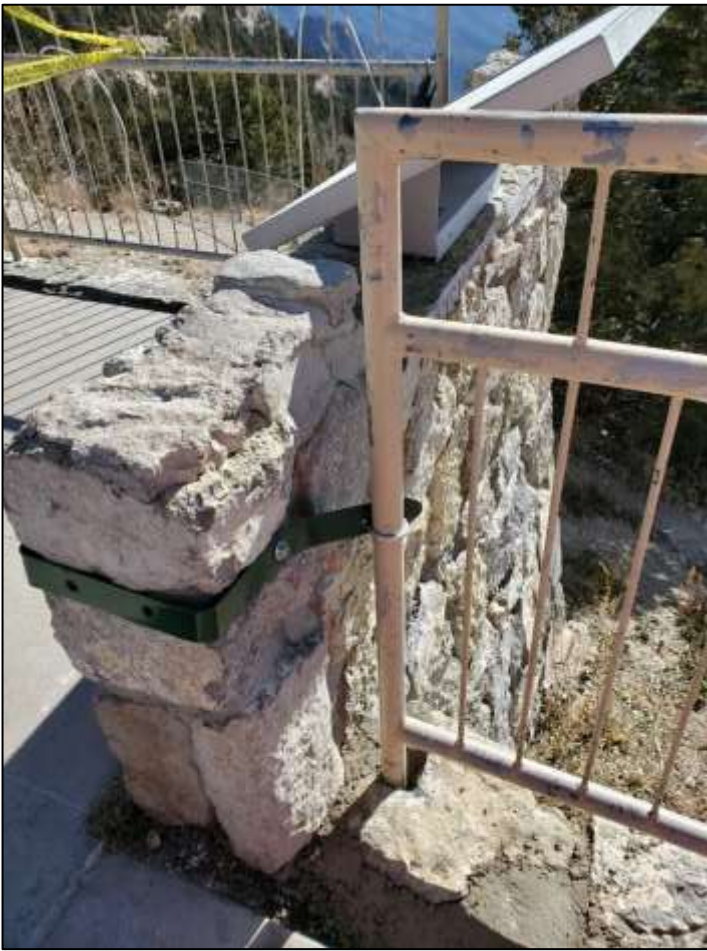
On the second work day, after the white adhesive material applied to the stone work in the previous photo was dry, the masonry was repaired, then some concrete was placed in the larger gaps.
