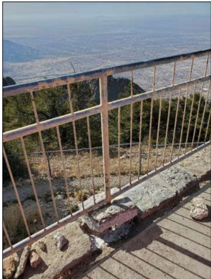
The middle post on the railing could not be braced very easily. Long ago a creative mason had drilled a hole through a chunk of limestone to help anchor it. Cleaning loose debris and applying the adhesive material required levitating the stone.
