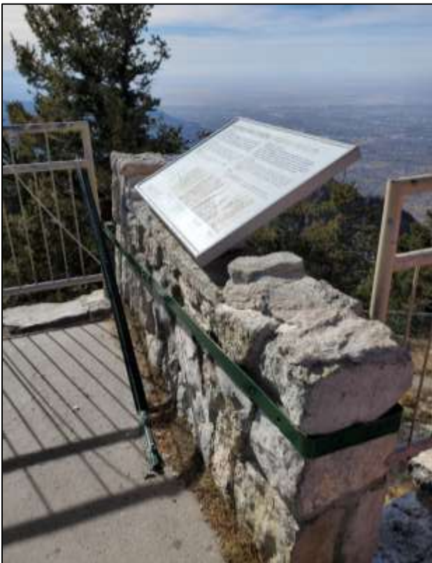
The post on the left side was not as easy and one of three possible options was implemented, securing the post to another railing on the observation deck which had been stabilized about three years ago by FOSM.
