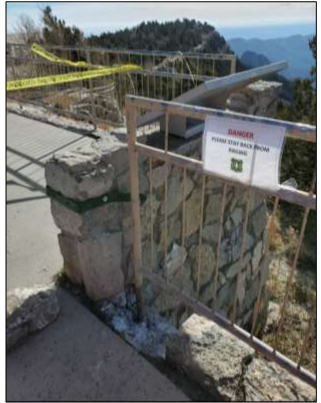
The steel band was wrapped around the wall and secured to the railing post. Then an anchor fastened the band to one of the mortar joints, luckily without breaking any more stones loose.
