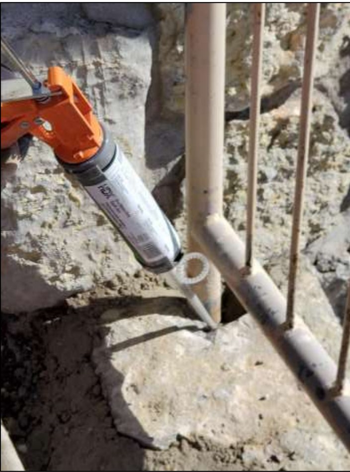
Finishing touch: anchoring epoxy was squeezed into the gap around the post. The epoxy does a great job of tying the post to the surrounding stone work.
