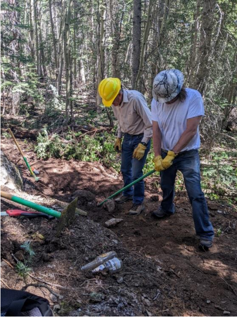
Michael and Sim take turns trying to pry out a rock. Don't bend the digging bar! After another attempt with a heftier rock bar, they decide sledging off the top will be a better tactic.
