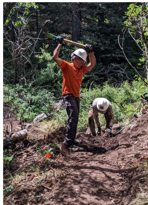
Luis goes after a root (must be) while Bruce works on the transition into the drainage
