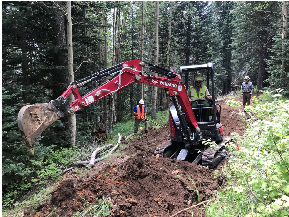
SRD Trails Foreman Russell Berman uses the horizontal blade on the mini excavator to smooth out the rough-cut left by the scoop bucket.
