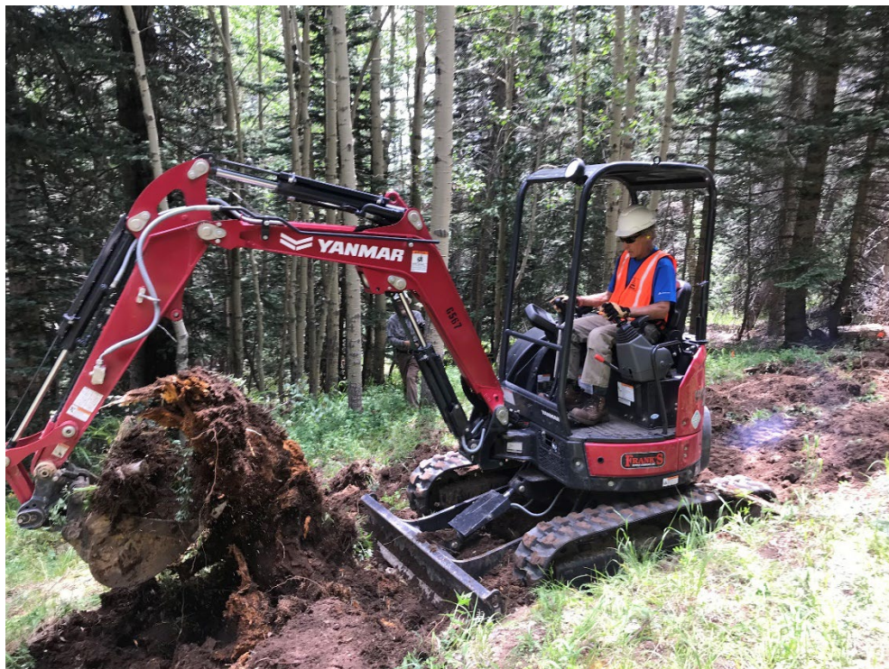
Jeff Huser using the mini excavator to dig out a large partially decayed stump.
