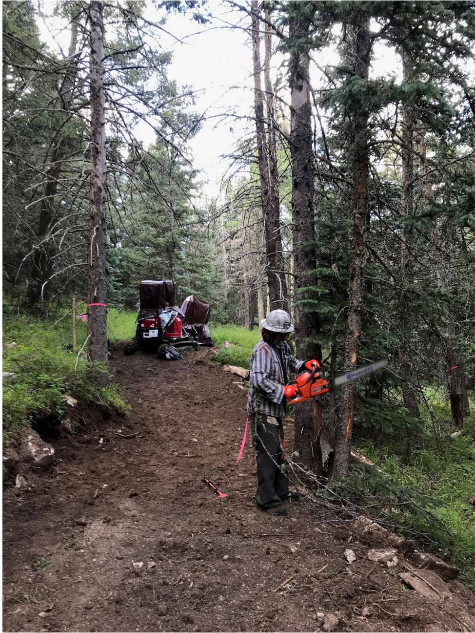
Michael Arndt limbing a small fir tree on the side of a section of the Klaus Trail which was recently graded with the mini excavator. This small fir, and the standing dead tree to its left were both felled after Michael completed the limbing prep work.
