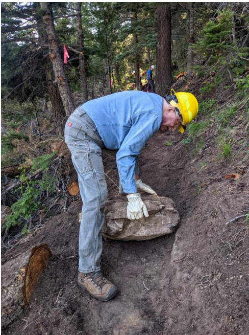
Sometimes the rock you need for cribbing resides downhill [insert Sisyphus comment here]
