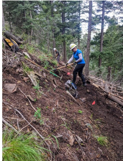
Courtnee and Luis prepare to do the same on a short section that needs rerouting
