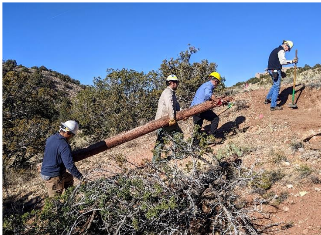
Jeff C, Russell, and Larry carry an unused piece of the bridge up to the old trenched trail. Jeff C then cut it into pieces which will be used as check-dams to slow down water crossing the new trail sections. Sim tamps a section of new trail.
