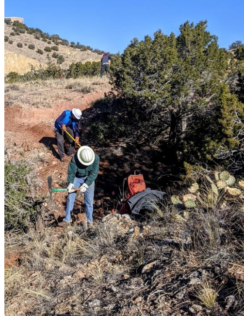
Byron starts a construction project across a drainage (behind him) (Scott, Tayo)
