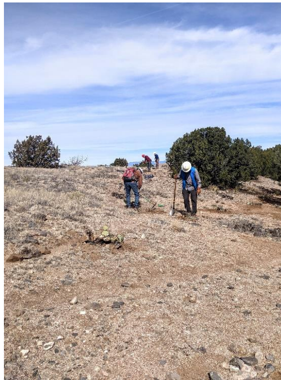
Criss-crossing user trails = plenty of work in this spot. Rocks come in handy.
