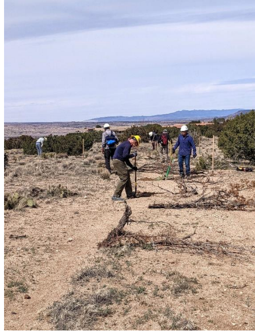
Still digging... The crew rounds out the day by completing the trail closure we started last month.
