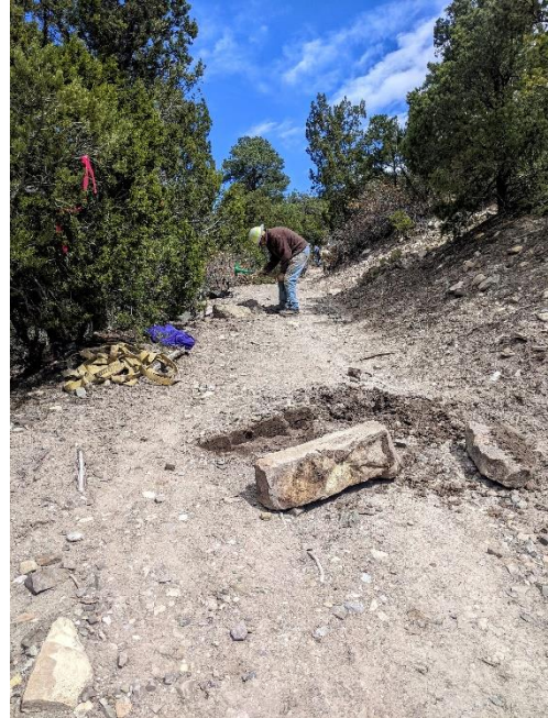
Jim extracts a rock for repairing the check-step in the foreground. (Good, this time the rock is uphill from the work.)
