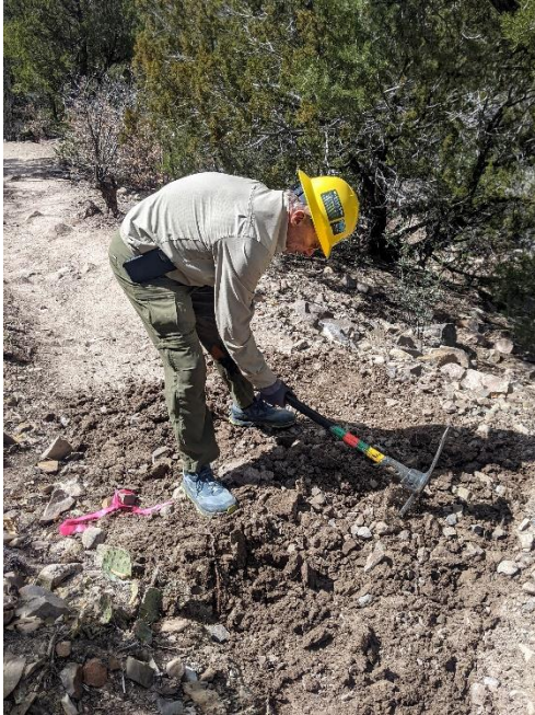
John breaks up compacted soil to put the dip in the drain dip
