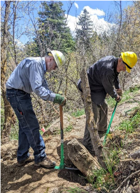
It's wiggling but they're not giggling. Cleve and Dan wonder just how long one rock can pretend it's coming out. (A second rock bar would have helped)
