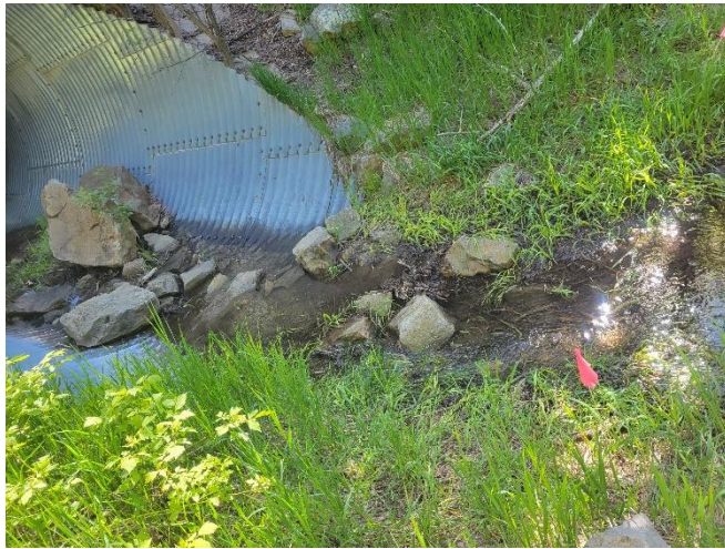
Bruce Hansche's before and after photos of the rock crossing ("after" taken during lunch ;)
