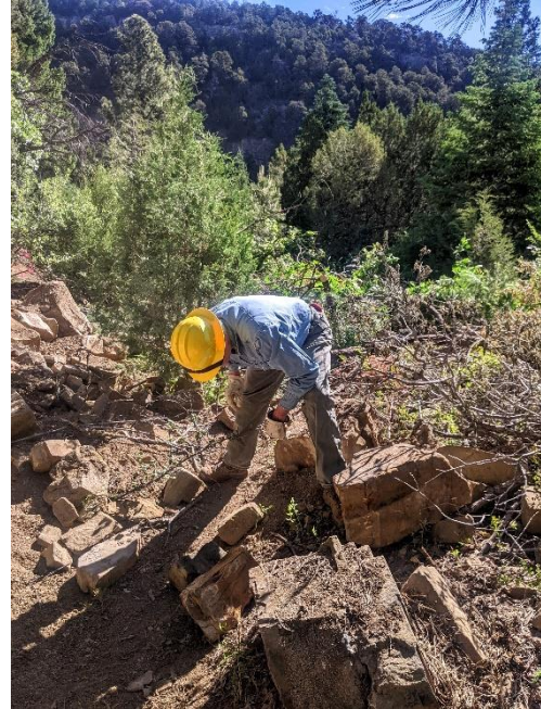
Eric goes low. Hmm, how to rubble it up without affecting drainage?
