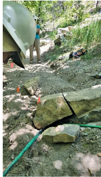
Photo by Luis Cuadros Luckily it had a crack
