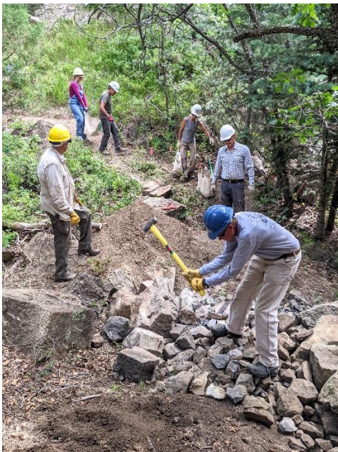
Work it Werkmeister! In the background Eve & Luis and Claudia keep the dirt coming.
