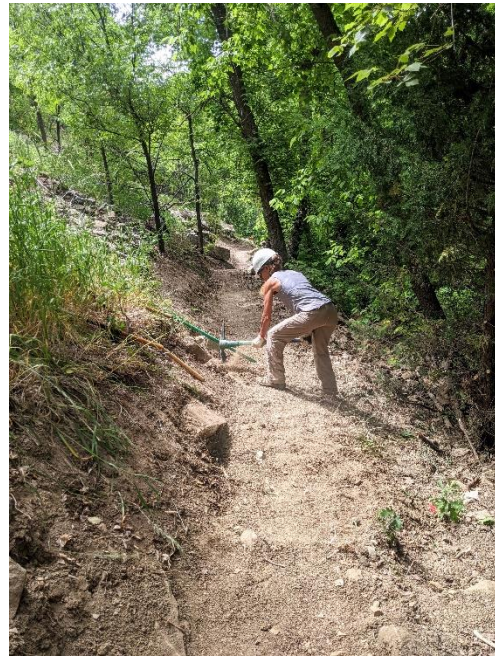
Claudia pulls out rocks near the backslope which could “push” traffic to the outside edge
