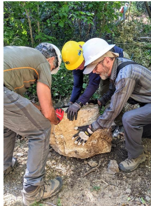
Luis, John and Bruce find a good one. Hmm, no rock sling on site today. They opt to roll it uphill.
