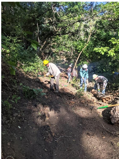
Dan, Tom, Jim and Claudia get started on the reroute. (John and Eric too, in the background/shade.) On the right side of the photo, the original line has been mostly closed off. Volunteers later finish closing it.
