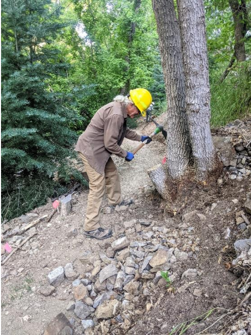
Mike removes loose debris from the backslope. Later Dan removes the stump.
