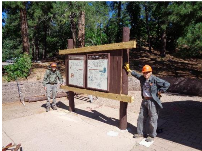
Sam Beard and Don Carnicom at the rebuilt kiosk at the first restroom in Doc Long Picnic Area. The new lumber was later painted with USFS brown paint.
