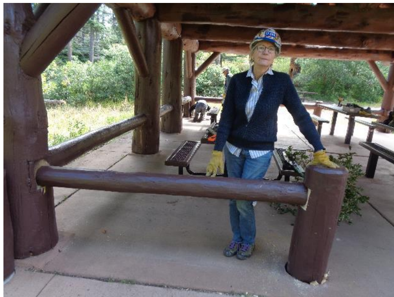
Joelle Hertel in the Balsam Glade Picnic Shelter where the post on the right and the horizontal beam were replaced after the original components failed due to decay
