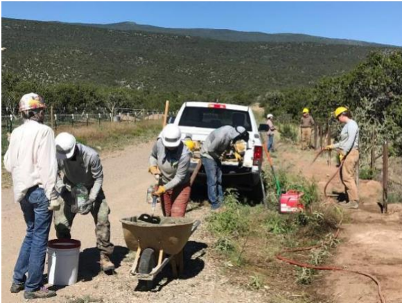
Activity along the west La Madera Gate pipe fence: filling gallon jug with water, mixing concrete, grinding rust off a steel pipe, spraying water on plants to reduce possibility of fire from welding
