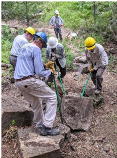
Mark Werkmeister, David Bernstein, and Dan Benton using rock bars to move a boulder to create a raised streambed crossing while Eric Russell works nearby
