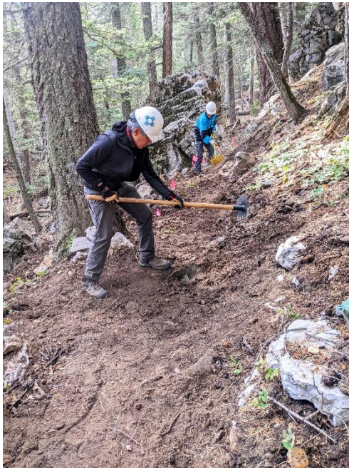
Meanwhile, Luis and Tony return to their benching project from last week.
