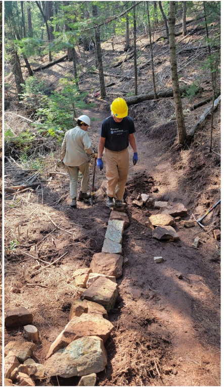
2 rows of large rocks are bedded on either side of the trail
