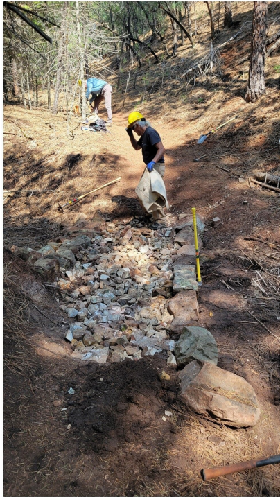
Rocks are used to fill the gap between the row of larger rocks then sledgehammered
