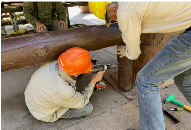
Installing a short post on Doc Long Picnic Area shelter, Don Carnicom and Sim Cook
