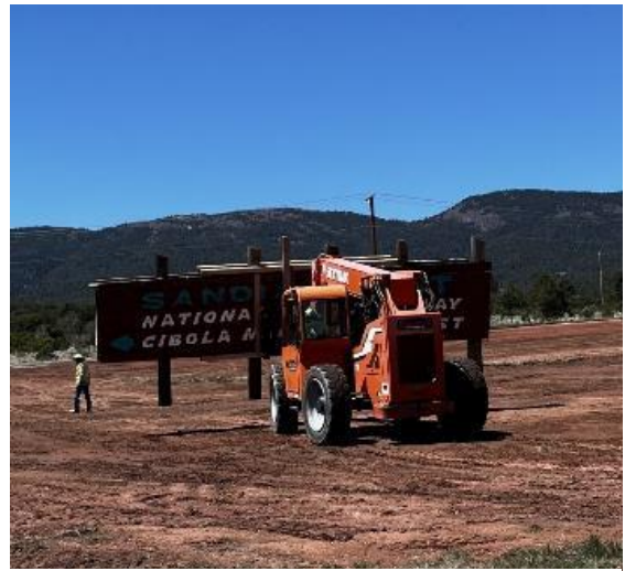
The historic Crest Highway sign being moved to the south-west side of the construction site
