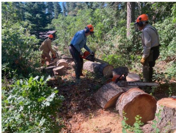
Sawyers bucking a felled hazard tree at the lower part of Balsam Glade Picnic Area. L to R: Dan Benton, Eric Russell and Sam Beard
