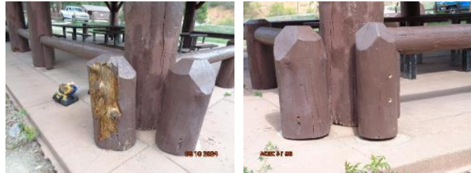
Before and after pictures of a replaced decorative post on a Doc Long Picnic Area shelter
