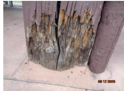
A decayed column base in Doc Long Picnic Area Shelter B
