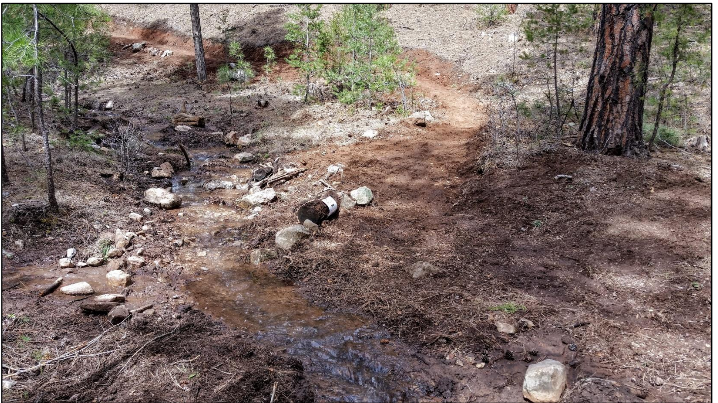
Bottom end of the reroute. One stream crossing then folks will be above the drainage, not down in it.
