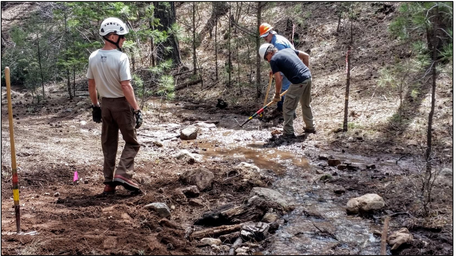
Ok, just couldn't keep the boys from playing in the water crossing at the lower end of the reroute...
