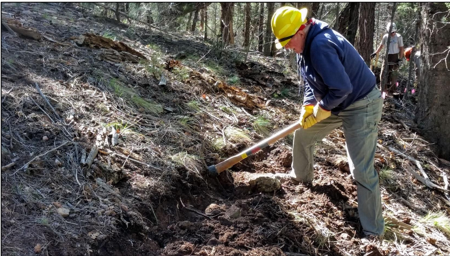
Toward the lower end, the sideslope got steeper and rocks started to appear.
