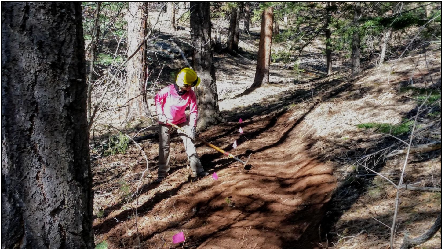
First task: apply finishing touches to the upper end of the reroute started last week.
