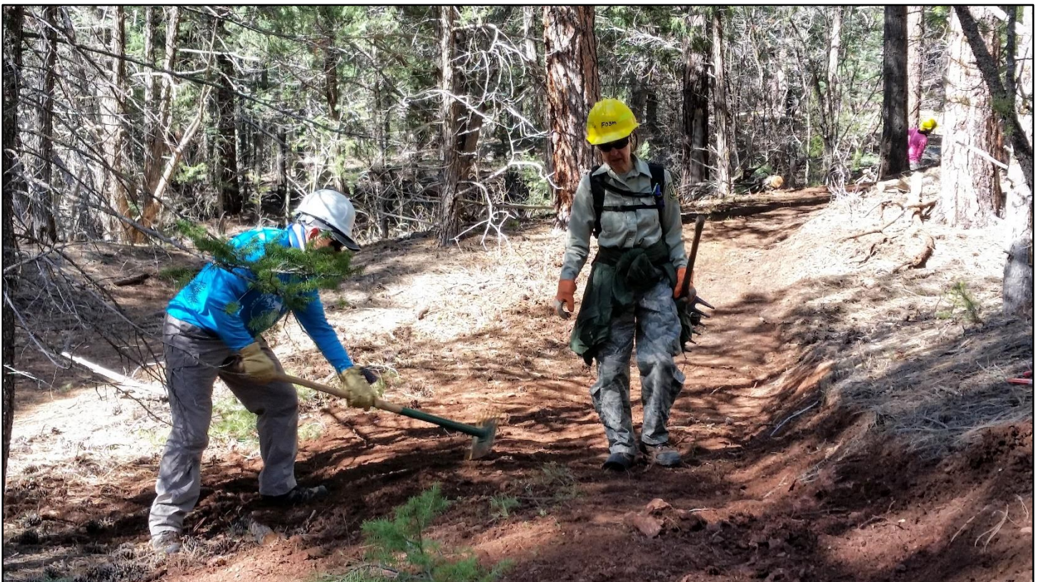
Cut the tread level, make sure the drainage works. This new line is a great improvement!
