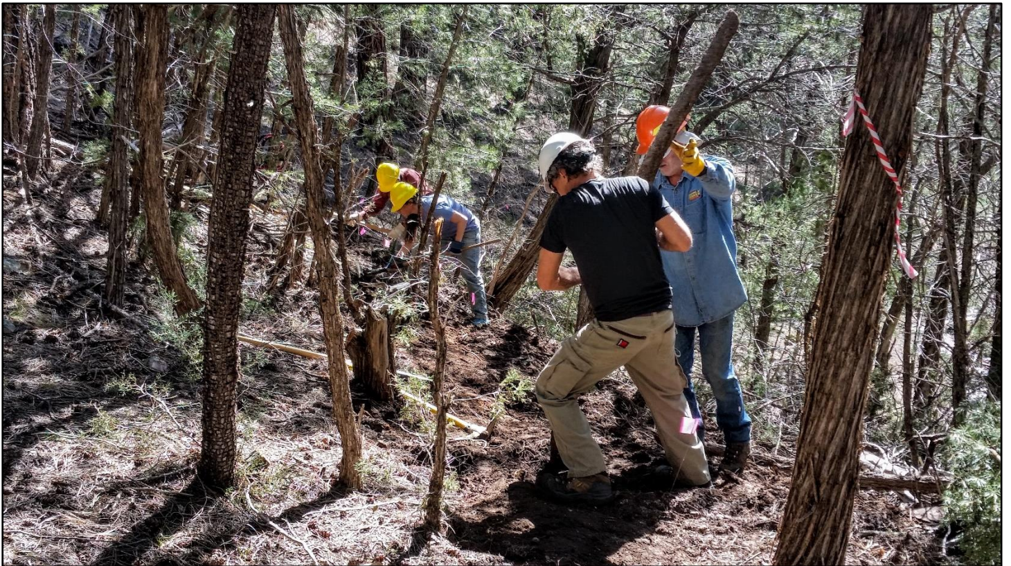
As the crew approaches the lower end of the reroute, there were plenty of stumps to pull.
