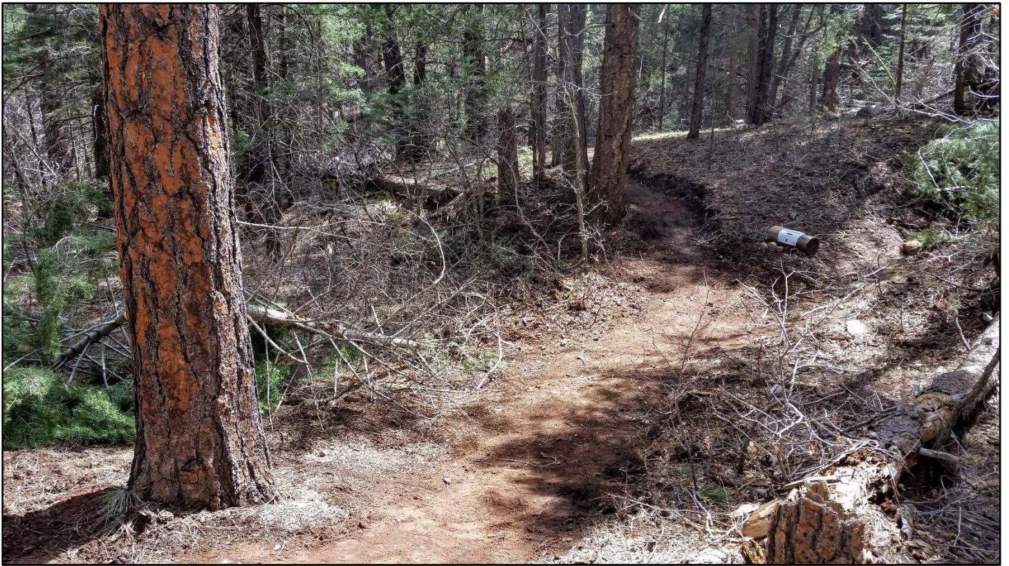
The top end of the reroute completed on April 4. The old trail section is now obliterated.
