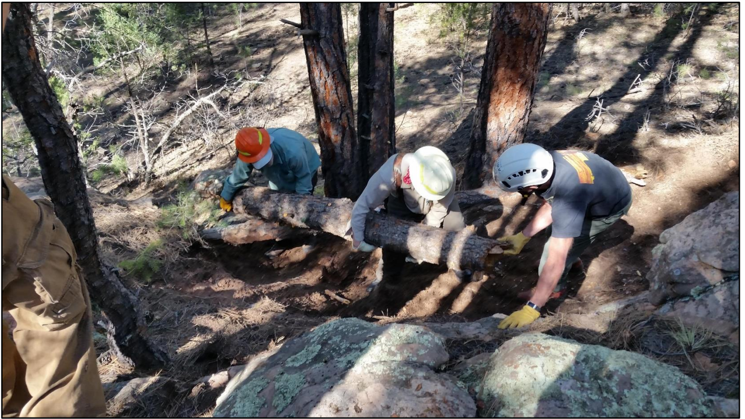
A temporary log retaining wall was cobbled together to control the boulder placement.
