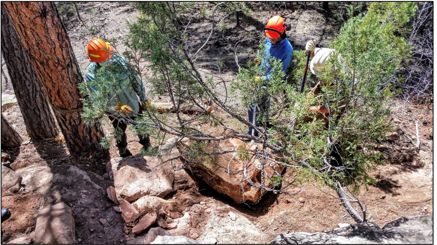
The last boulder keyed right in. But much coaxing was needed until it found its final resting place.
