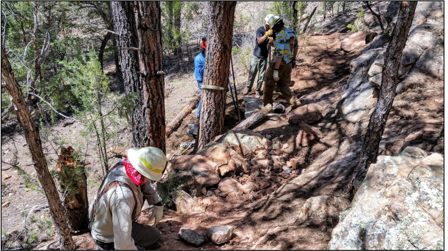
With the upper crib wall complete, some serious backfill was needed to fill the void.
