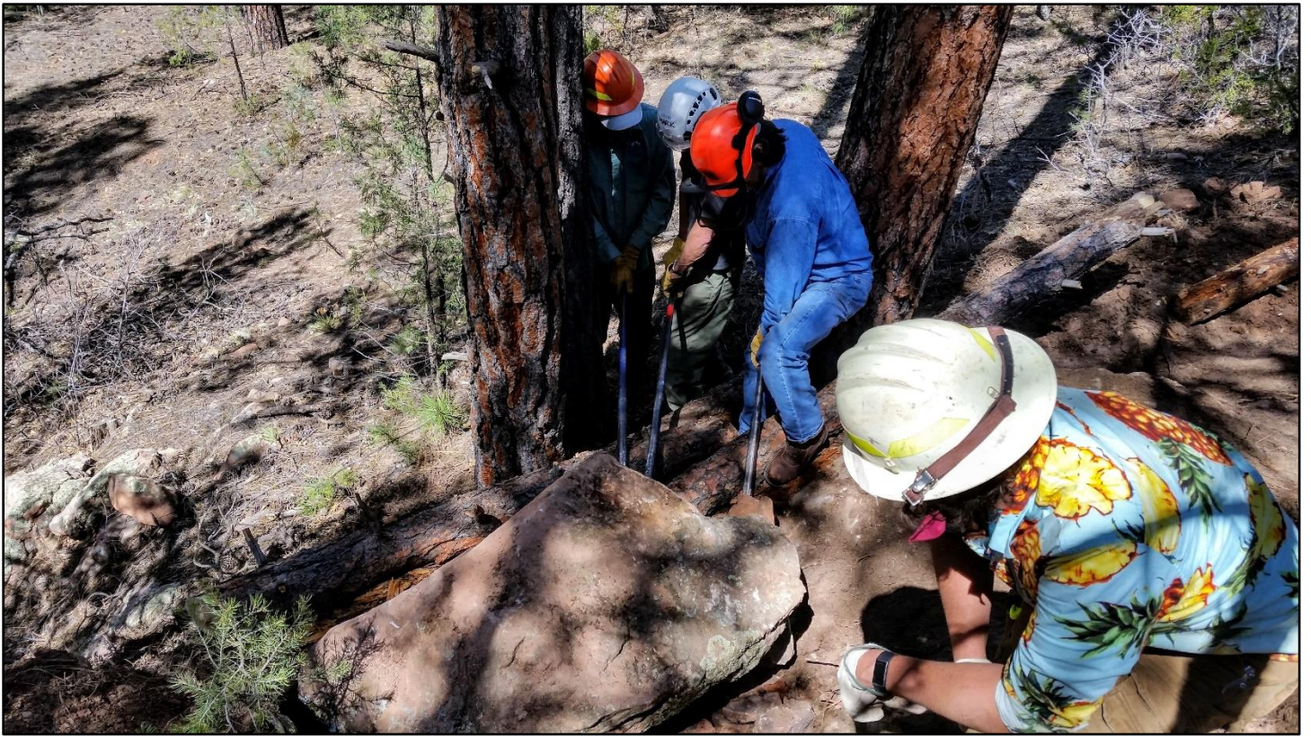
Ok, now to position it. Three rock bars were used to move the rock right where the boss wanted it.
