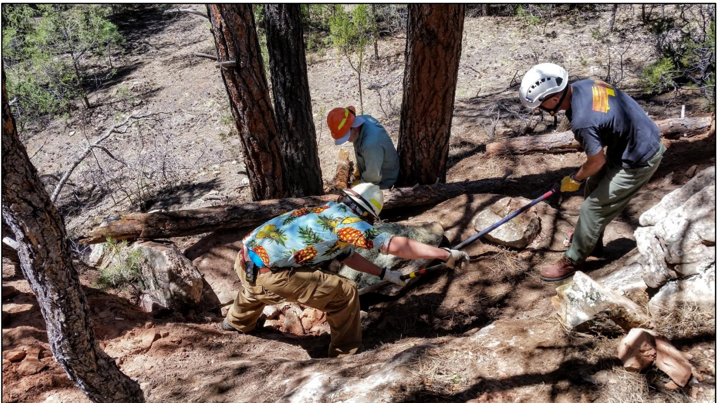
With the big guy in place, other boulders were moved in to complete the crib wall.
