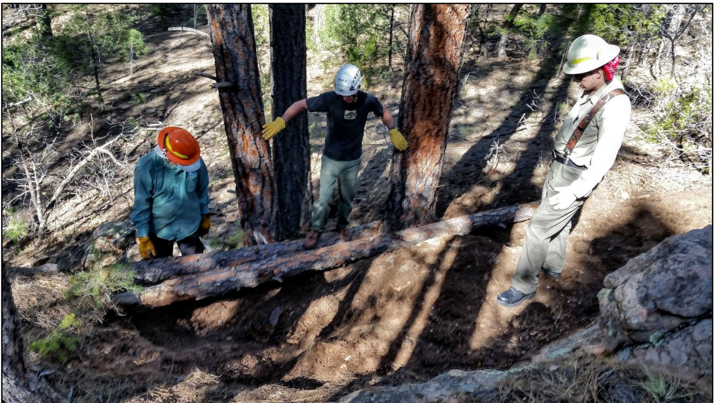
Ok, that boulder is pretty big and this log retaining wall looks really feeble, but it is what it is...
