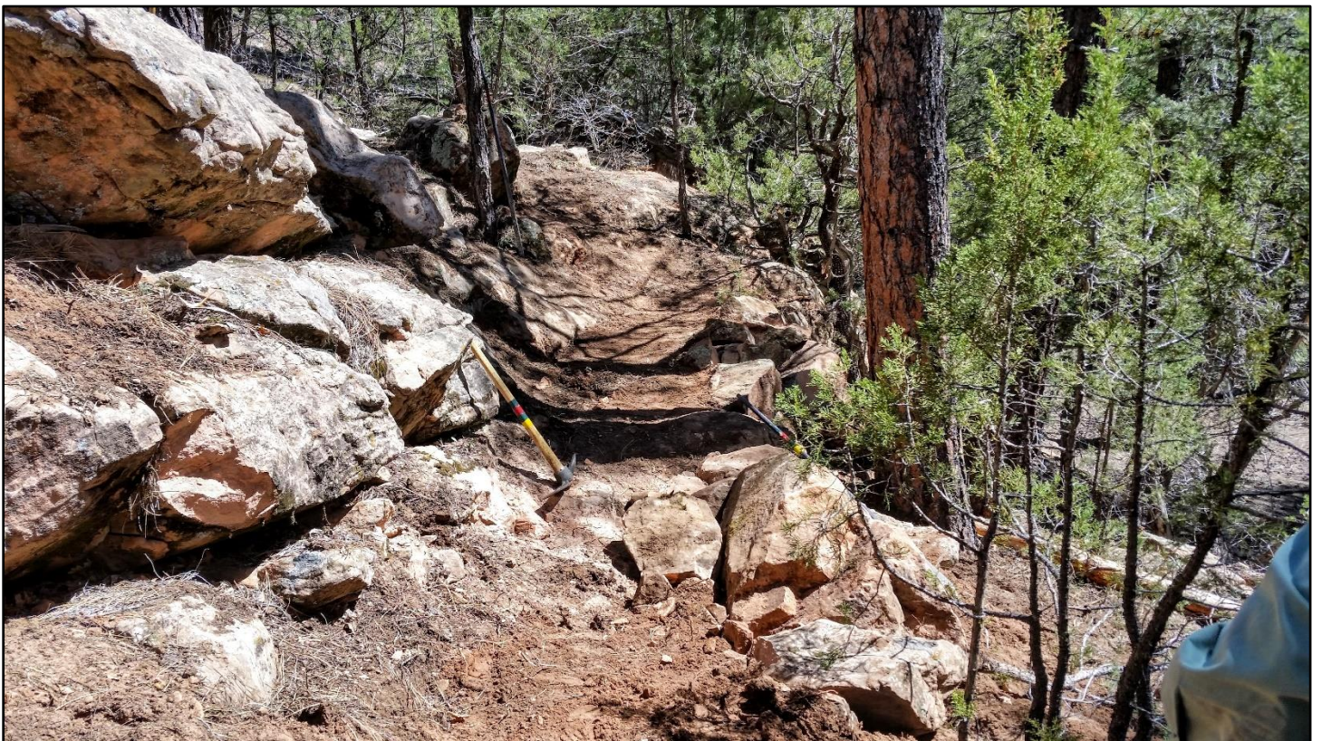
Crib walls are complete but more backfill is needed. We closed the section until we can get back to it.
