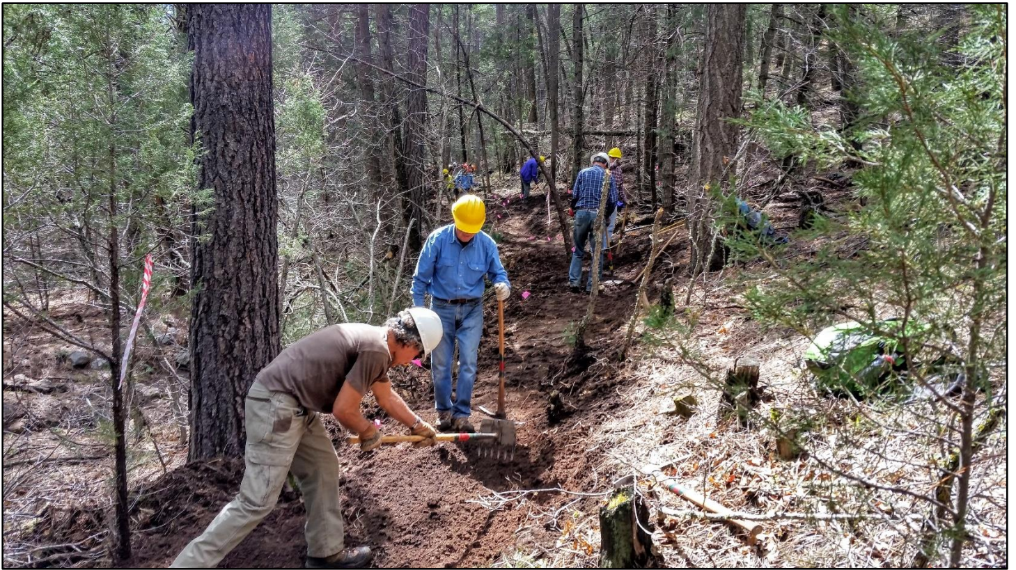
The experienced FOSM crew cuts in the tread. Soil conditions were perfect for building trail.
