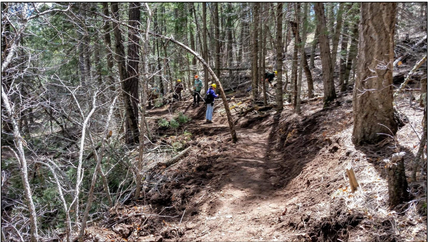
The tread is finished here. We're not yet connected but trail users will prefer the improved line.
