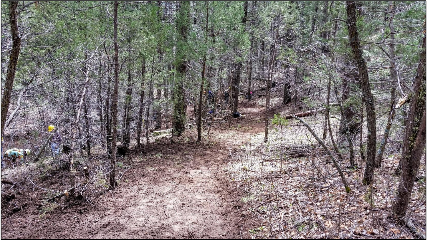
A new section of TC24 winds up the ridge. More sustainable than the fall line user trail it replaces.
