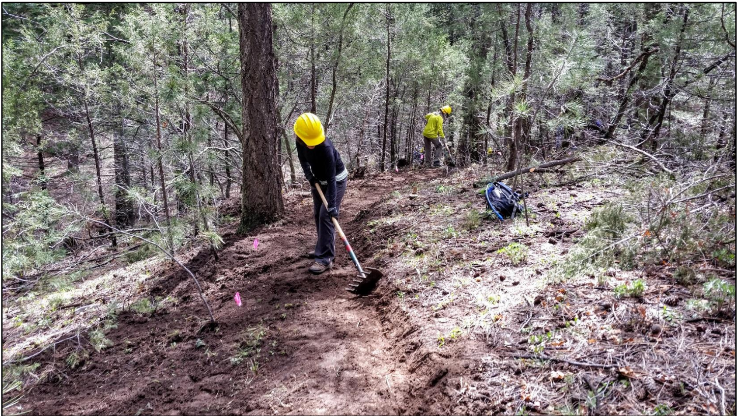
After the Mayhem and Destruction Crew plows through, this team brings the trail up to standards.
