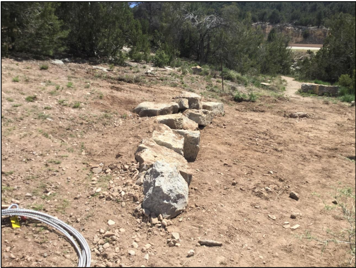
At Ranger Rock, a new retaining wall was completed to back up the future informational kiosk.
