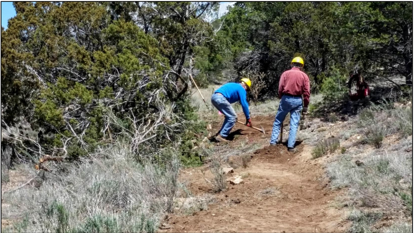
The final few feet of tread are cut in at the upper end.
