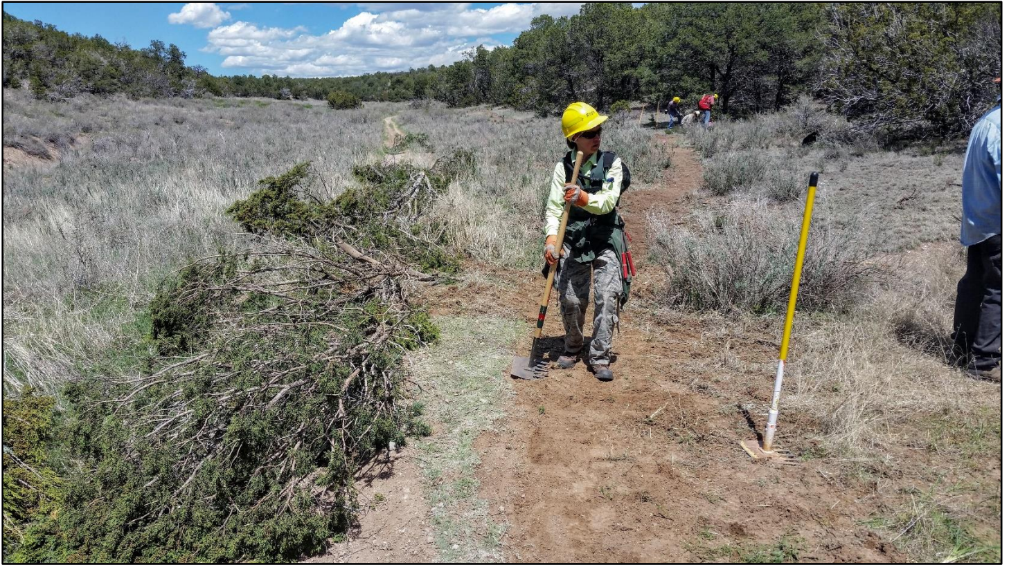
The lower connection is tied in and slash was dragged onto the old trail to discourage use.
