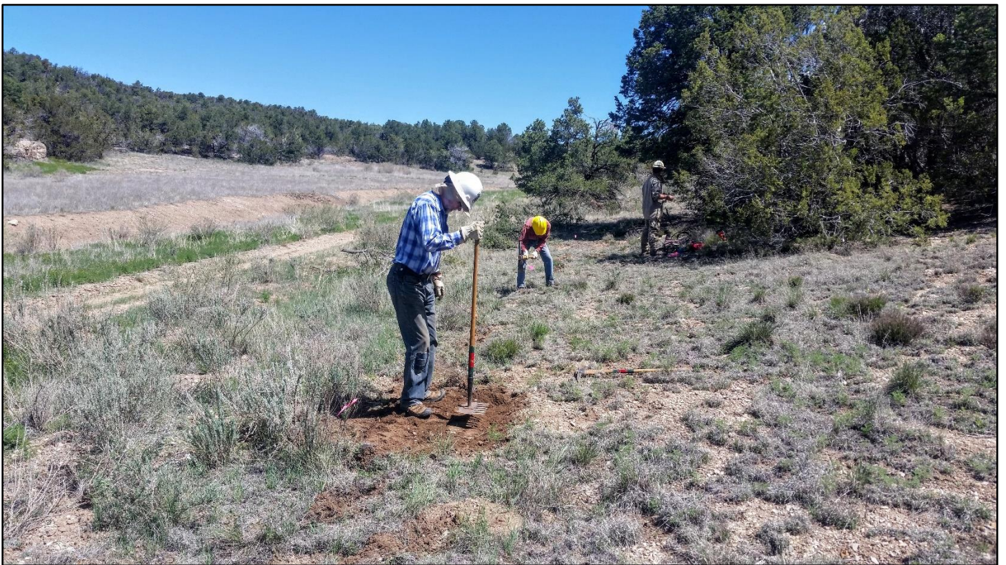
One gets a sense of accomplishment cutting out and finishing a section of tread.
