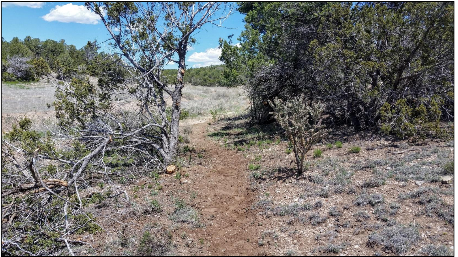
The upper connection is tied in. This connection is temporary until the line is extended up the canyon.
