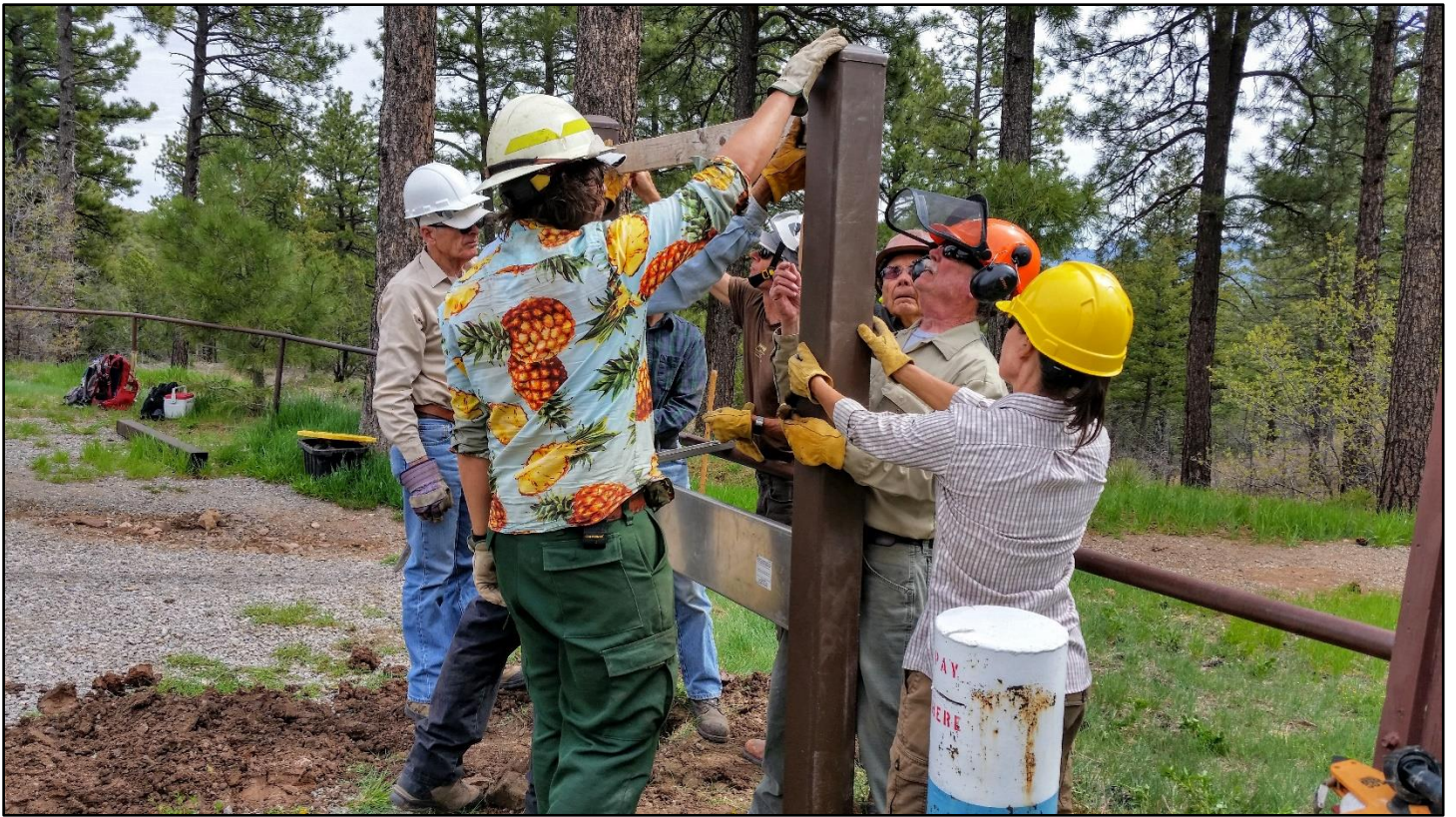
Now we're making progress. Install the templates and keep checking with that level.
