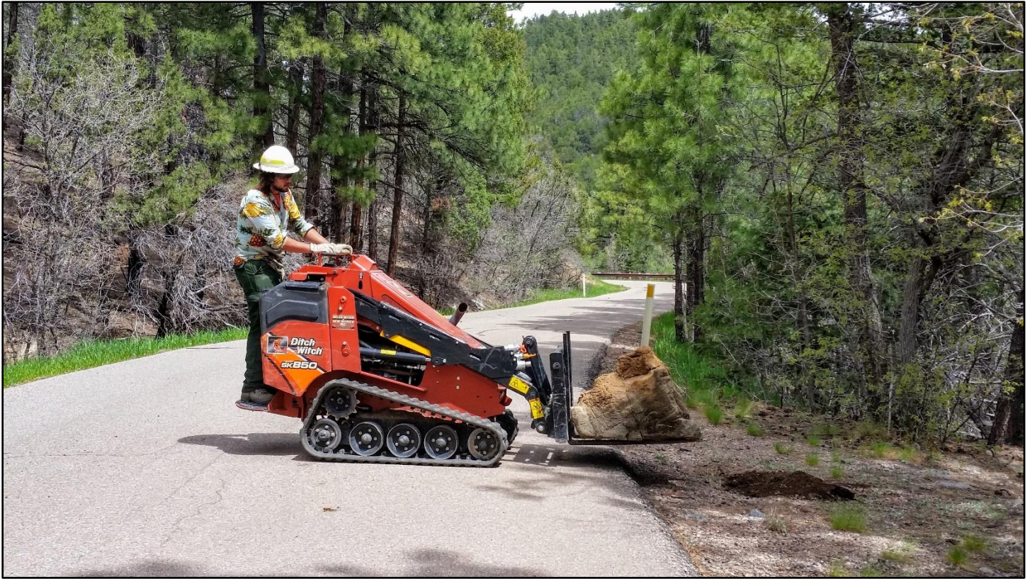
Final task: A few well-placed boulders will discourage random parking near the road.
