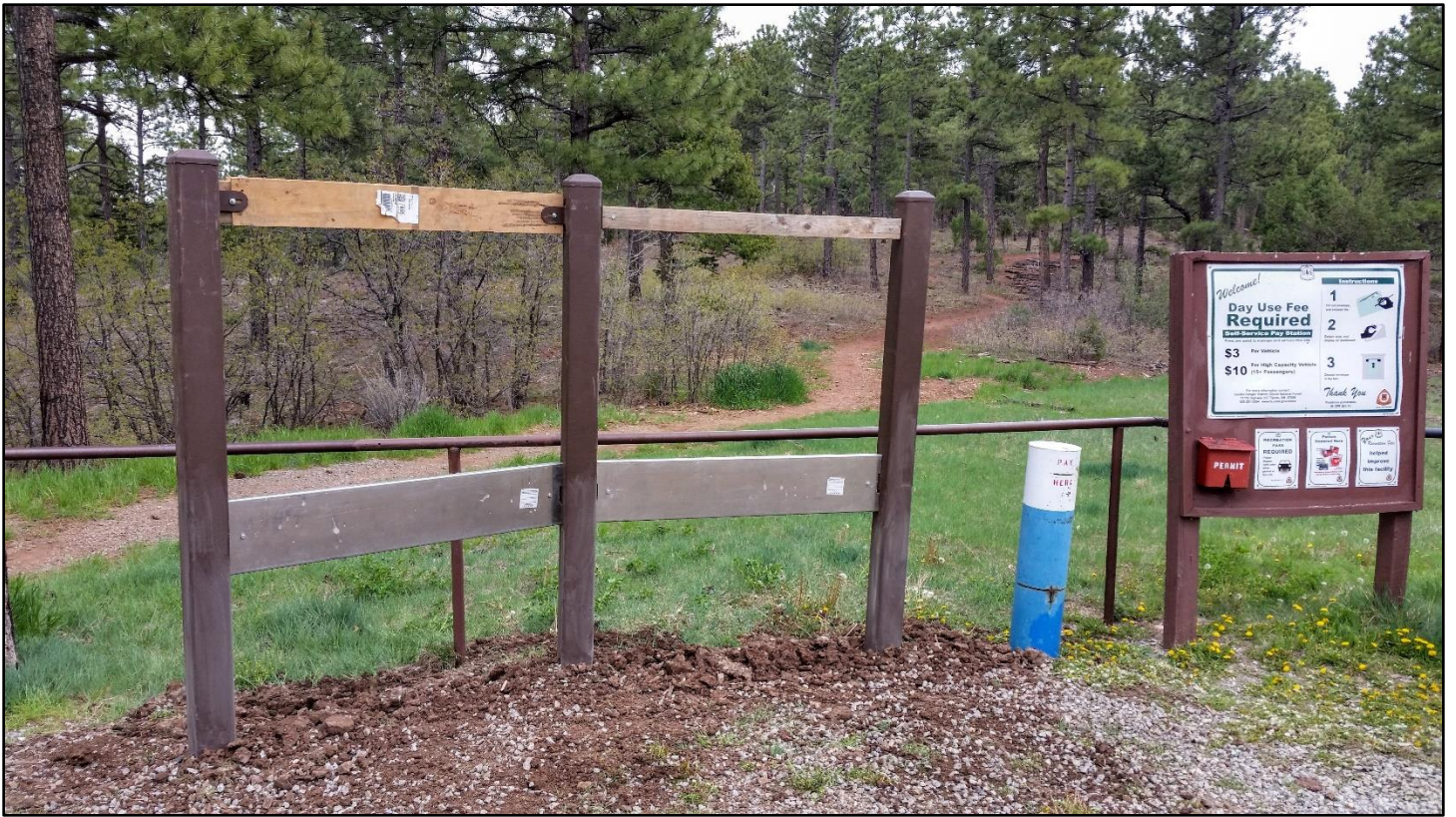
After: The templates come off, the panels will be installed, and the REI-provided kiosk will be finished.
