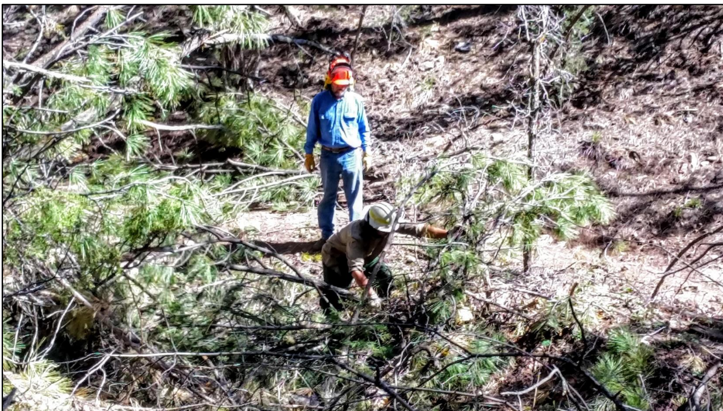
With the longer reroute nearing completion, obliteration progresses on the bypassed section of trail.
