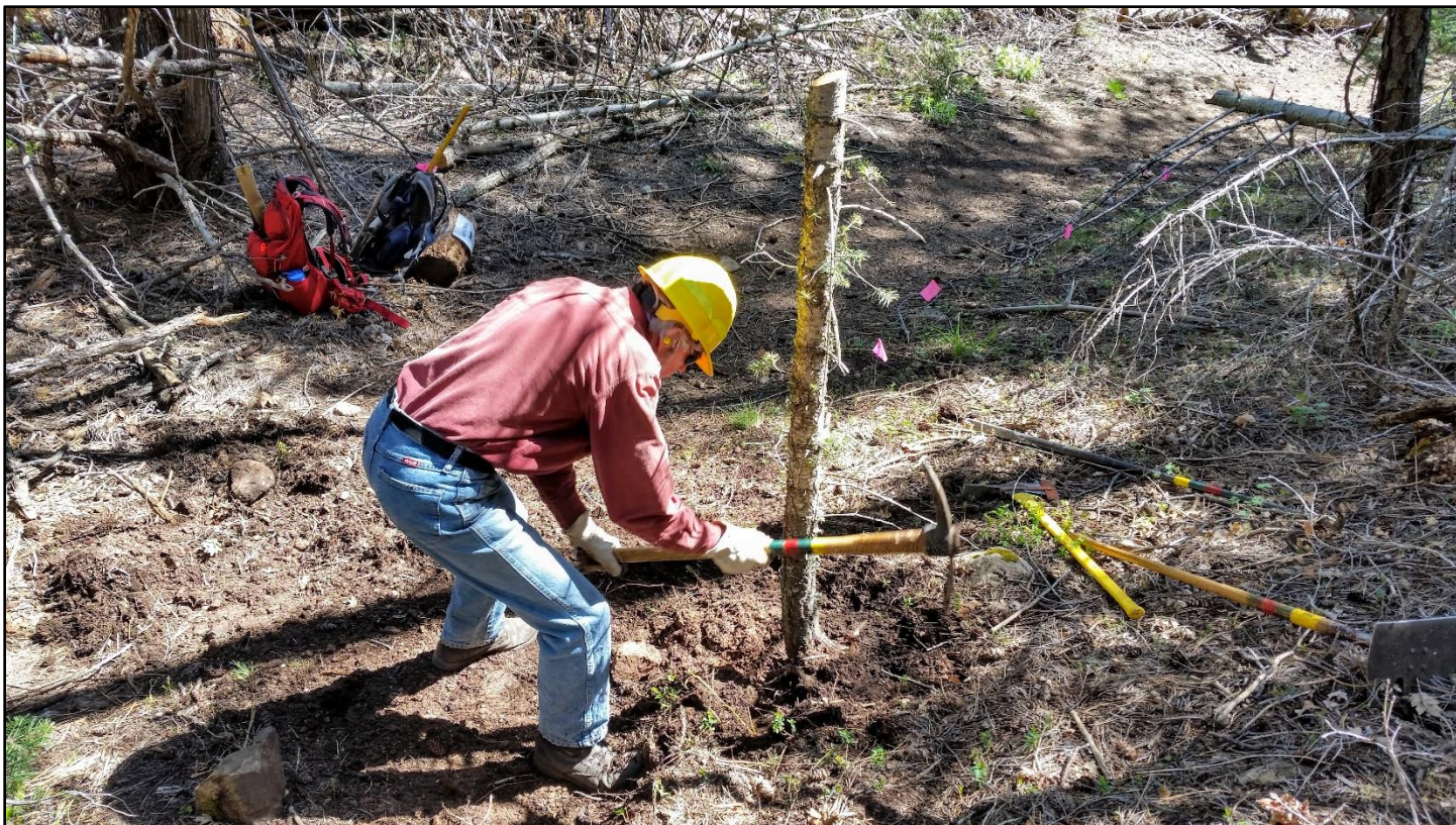
Digging out a stump to merge the lower end of the longest Armijo reroute into the existing trail.
