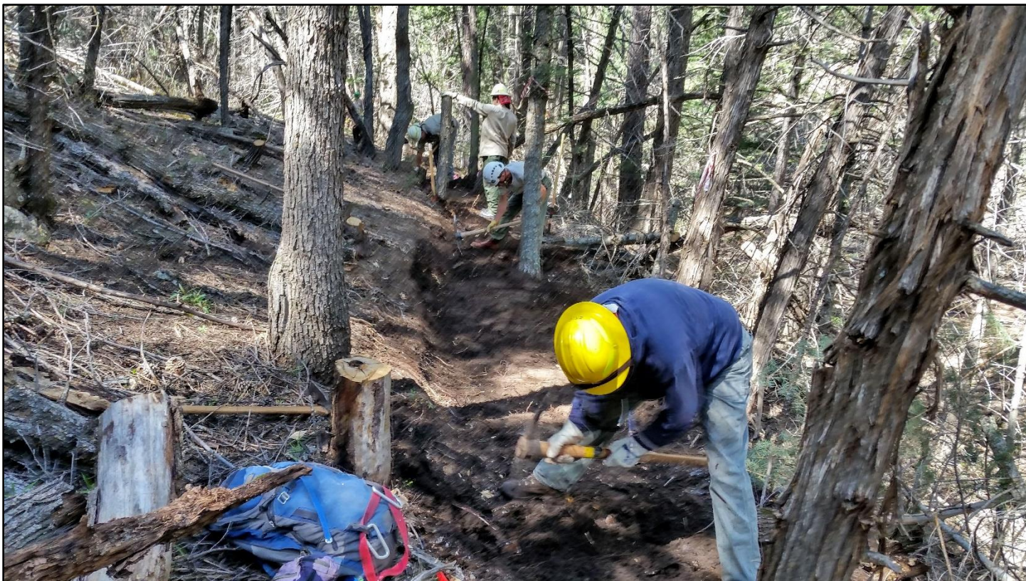
At the lower end of the reroute, heavy duty trail work was needed to cut in the new tread.
