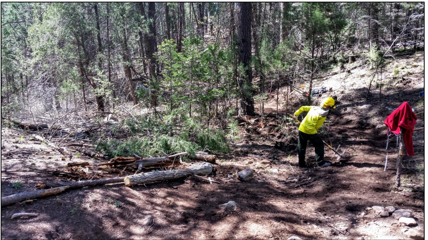
Upper connection of this Armijo reroute gets finishing touches. The bypassed section is obliterated.
