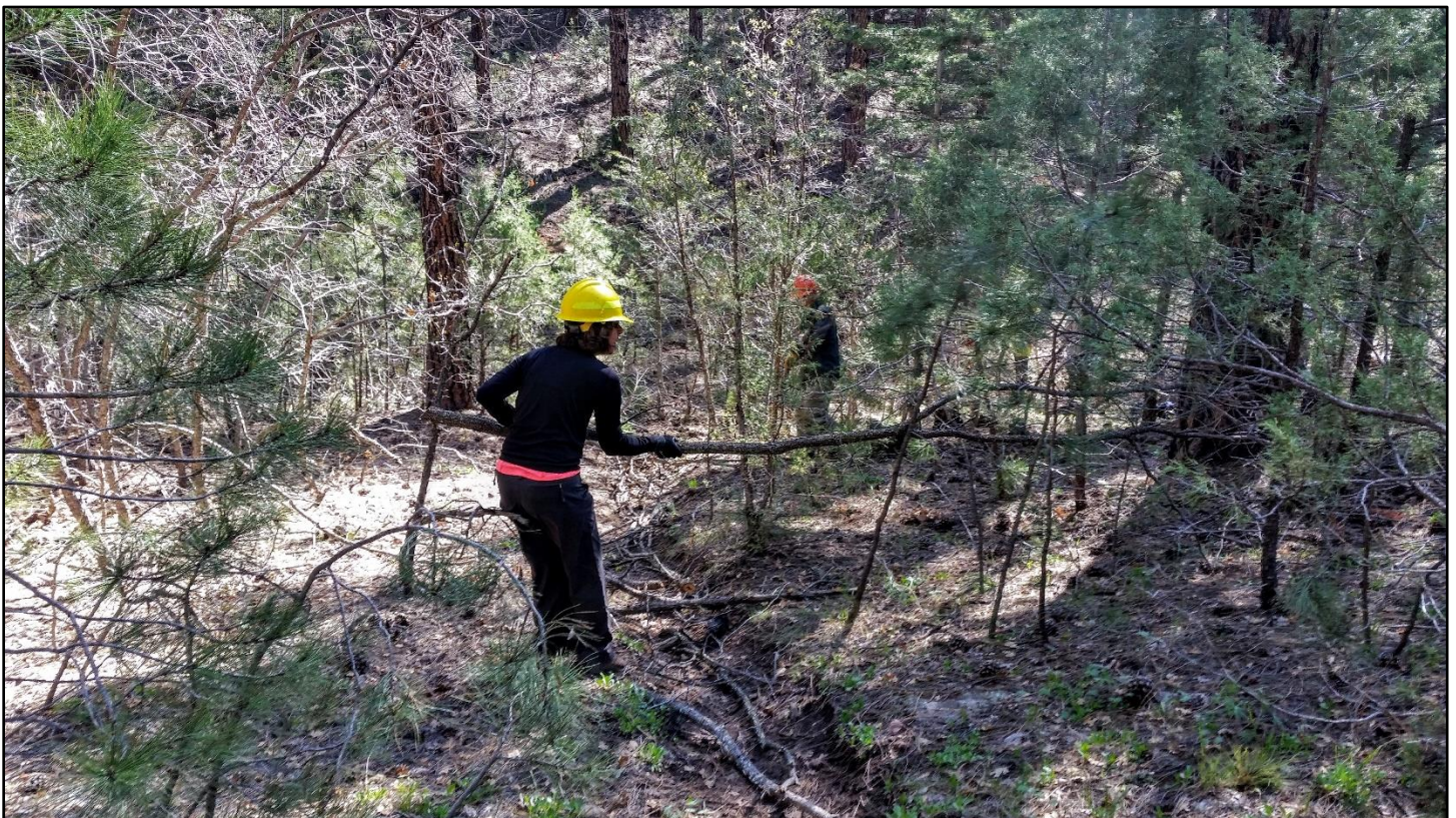
With the first CATIP TC24 connection complete, the crew obliterates the fall line user trail to Armijo.
