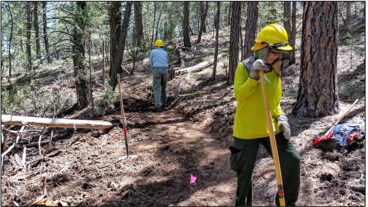
With the work on Armijo winding up, part of the crew moved up to a reroute of CATIP TC24.
