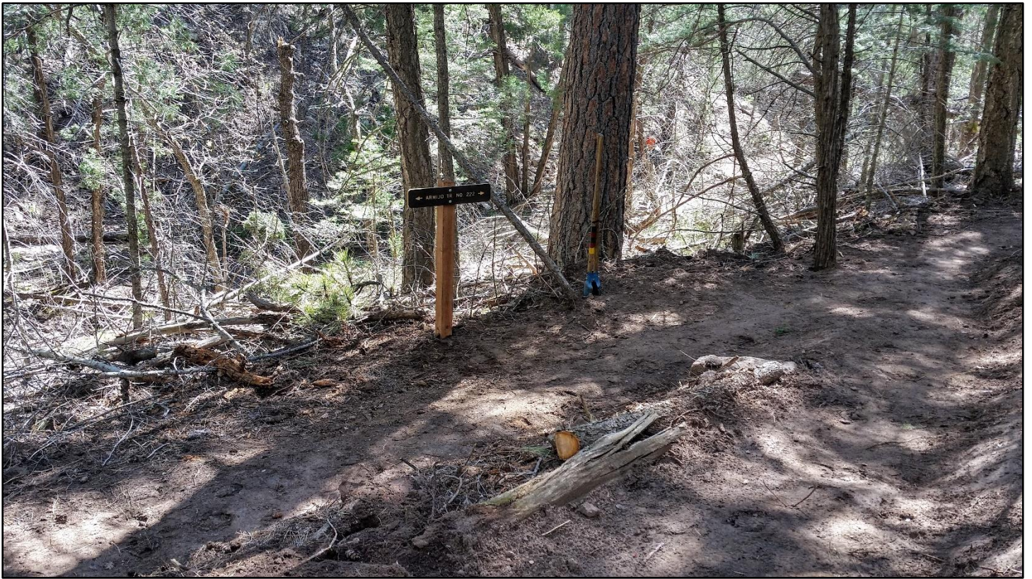
The crew even installed another REI-provided trail sign at the junction of Armijo and CATIP TC24.
