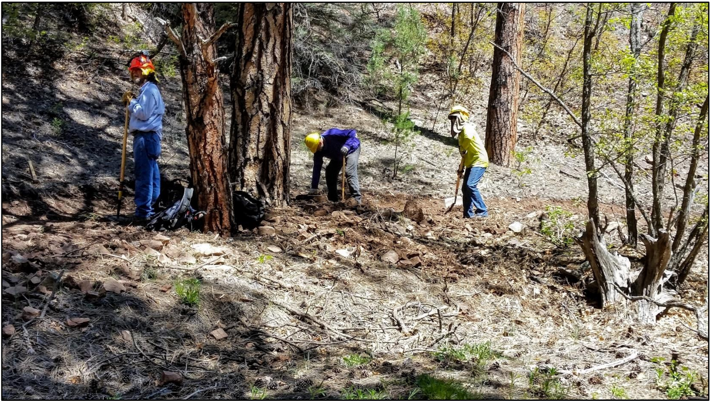
Widening the trail around a large ponderosa turned out to be quite a job in the rocky soil.
