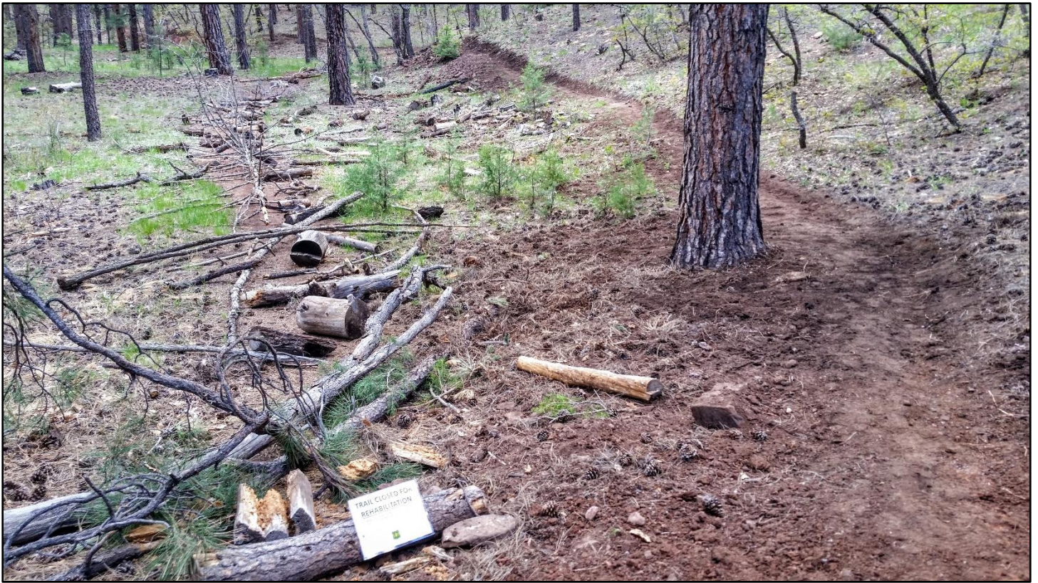
The lower end of the reroute is cut in and the old trail obliterated. The trail is now out of the drainage.
