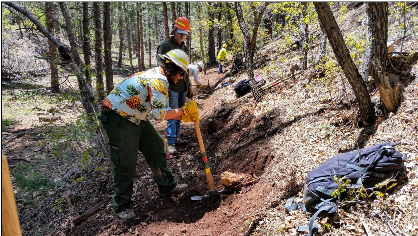
Two oak stumps were just too close to the trail but took some persuasion to cut out.
