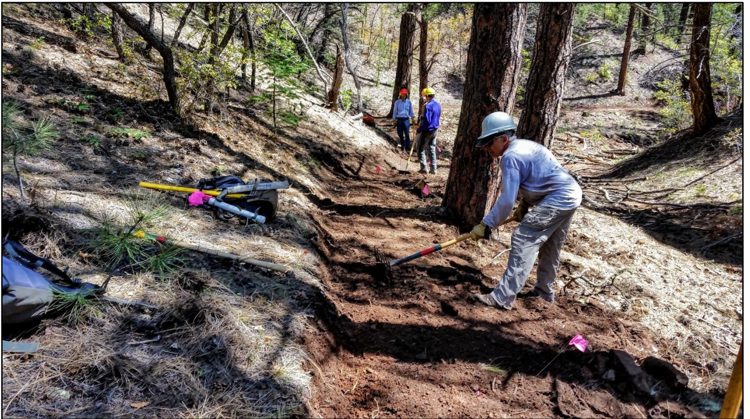
A lot of the effort today was cutting the tread level: easier to walk on, better sustainability.
