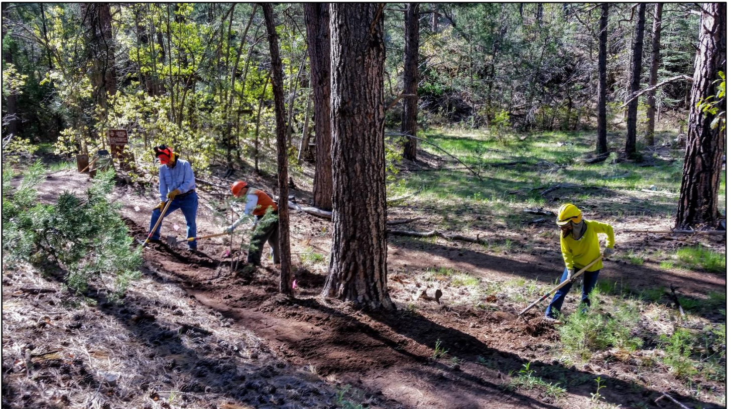
Part of the crew starts to cut in the lower end of this Armijo Trail reroute started last December.
