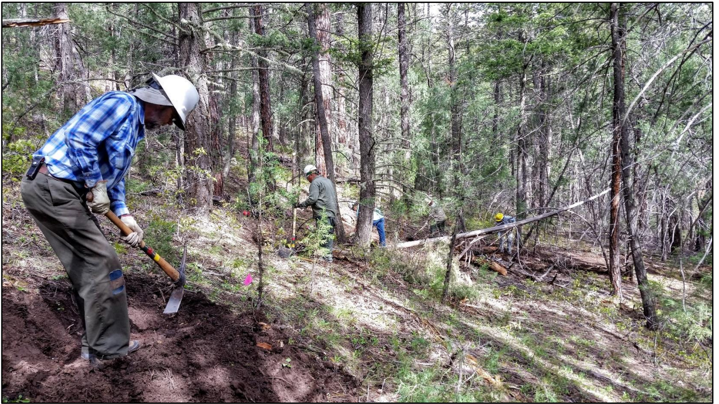
The crew is hard at it on the reroute. The soil is still almost muddy in places.
