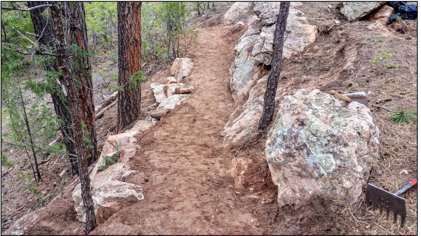
Boom, done! The crew completed a very nice section up the rock outcrop.
