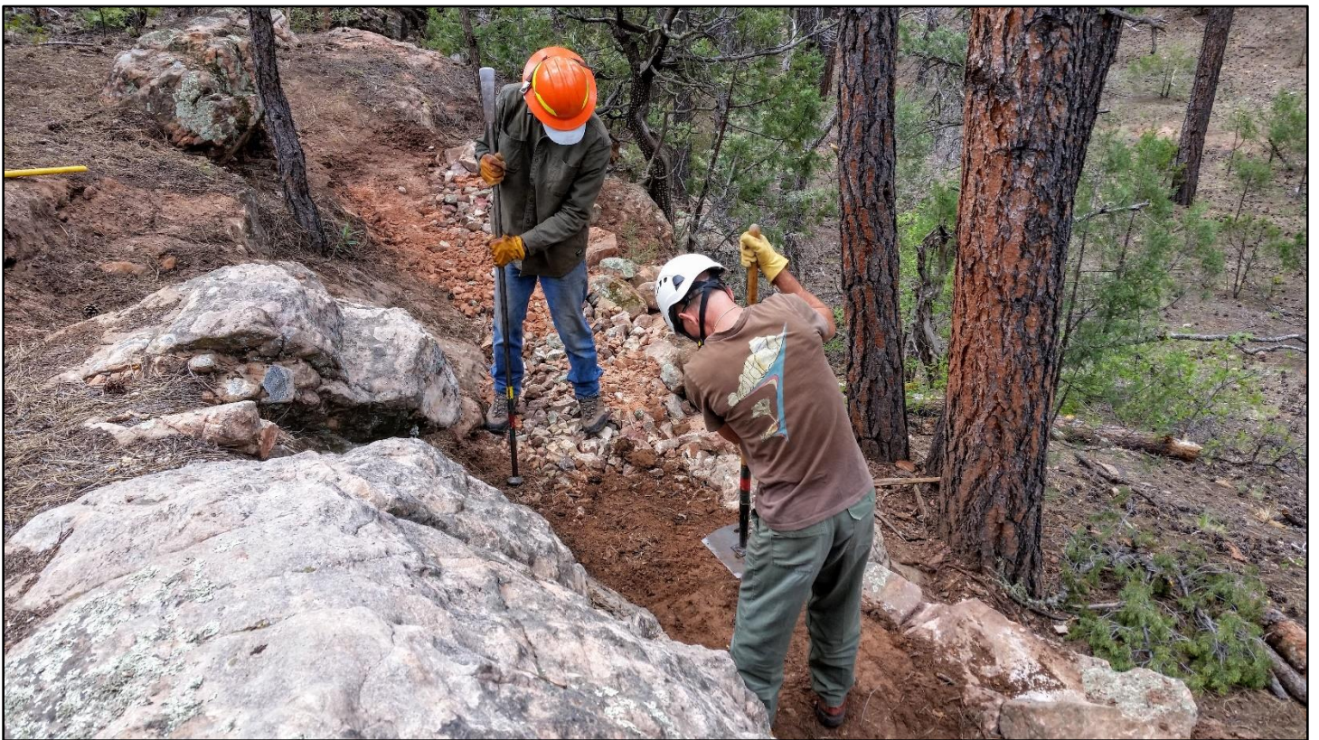
After a lot of rock backfill and a lot of rock crushing, the top layer of soil comes in and gets tamped.
