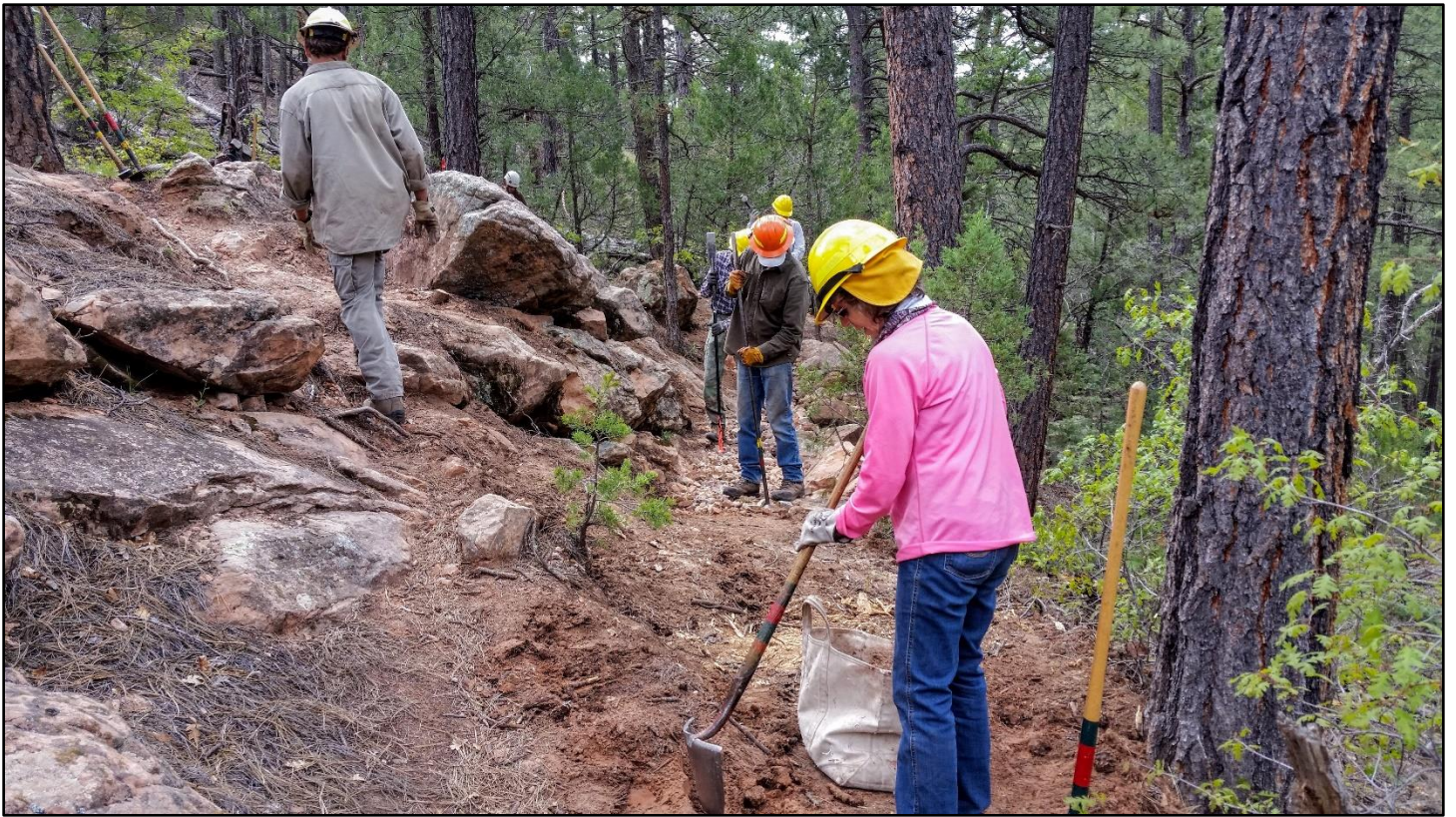
The rock crushers get with it, the dirt crew finds dirt, and the chain gang boss keeps an eye on things.
