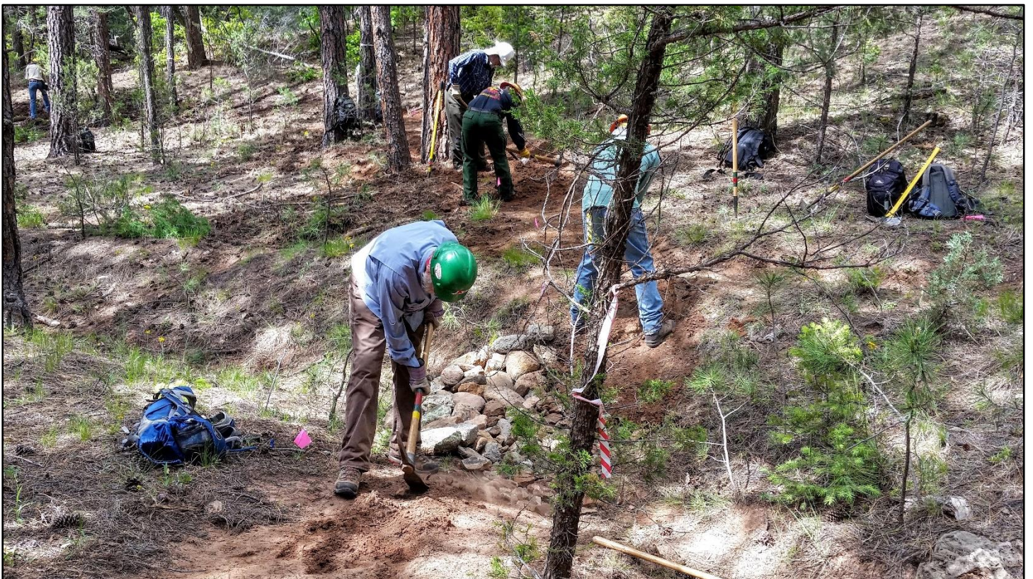
Dirt is pulled down on a drainage crossing which has been backfilled with cobble.
