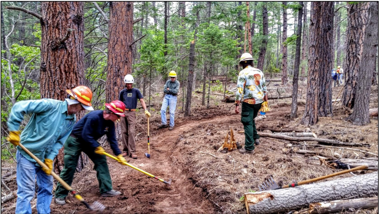
Finishing the lower end of the reroute. The boss was surprised we finished the entire section.
