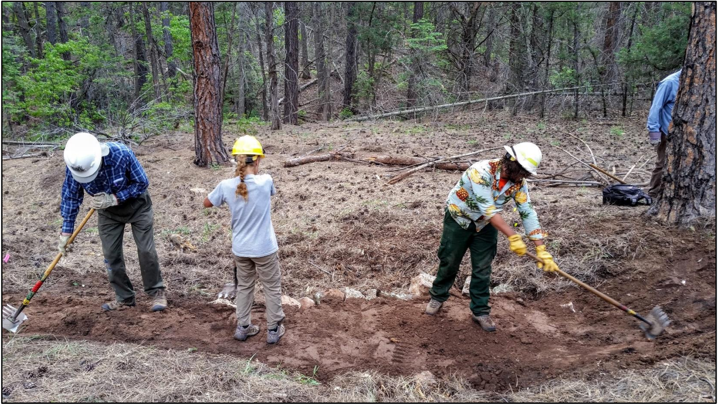
Done. Dirt is dragged in to complete the crossing. And we saw it hold up well to the three equestrians.
