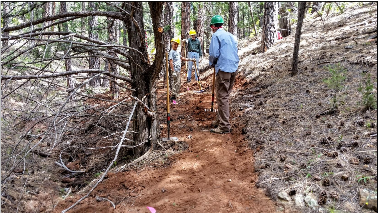
At the lower end of the tough section, extra dirt had to be requisitioned to finish the drainage backfill.
