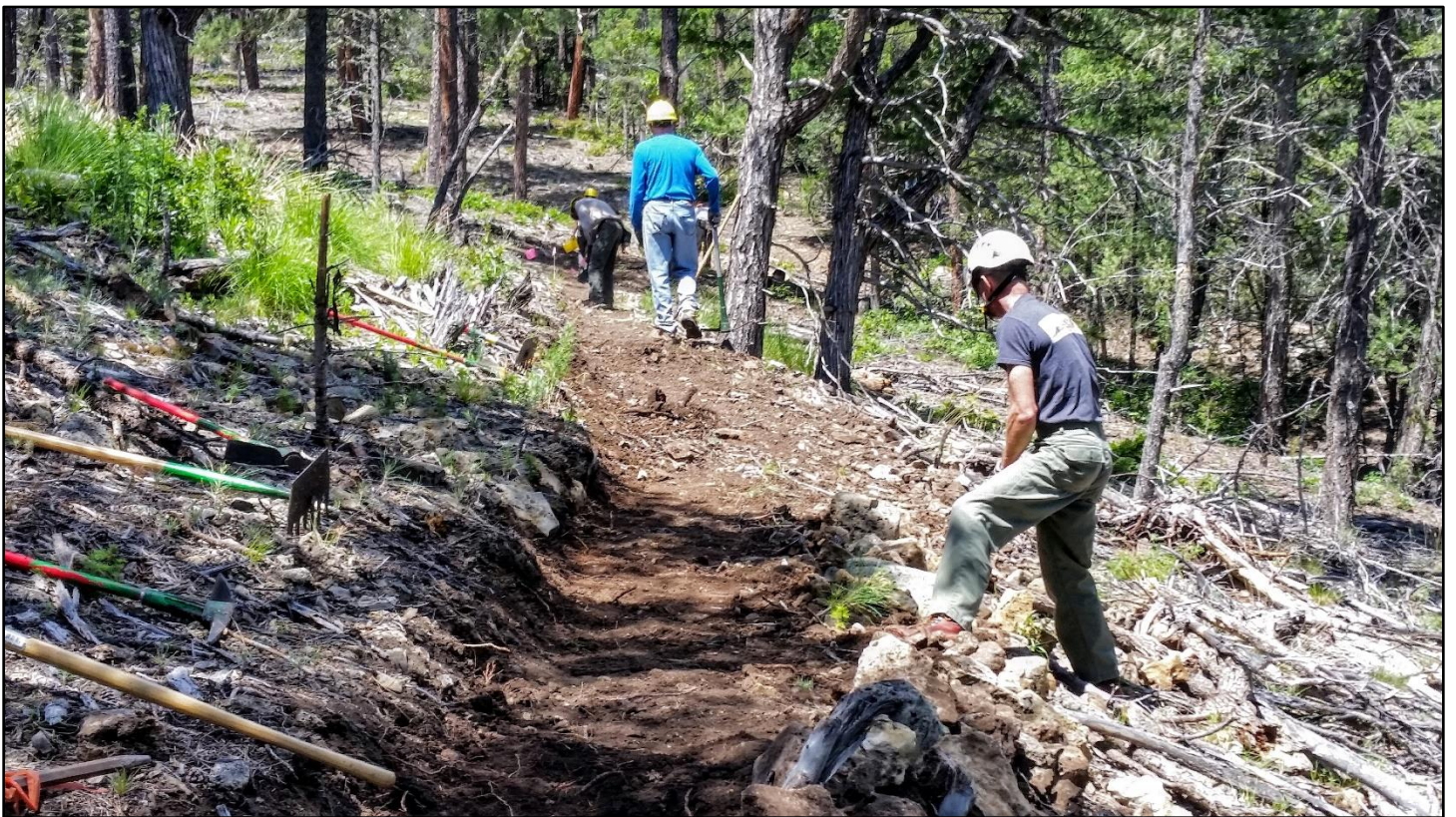
Boom, done. Nice wide, level trail. A LOT of rock was pulled out to level the tread here.
