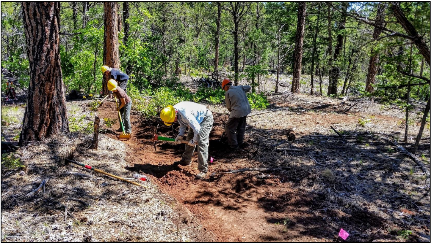
The crew cuts new tread toward the lower connection. The bypassed user trail is in the background.
