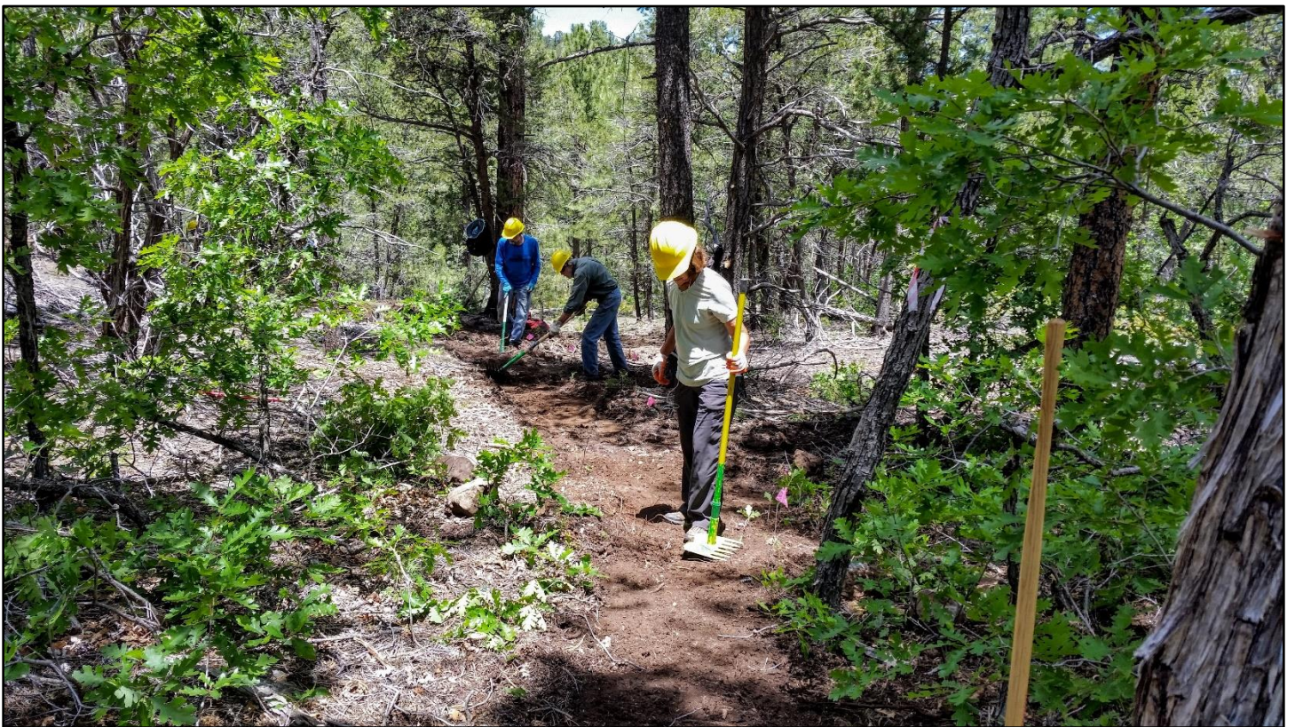
The crew works their way towards the bottom of the canyon. The gambel oak is thriving this spring.
