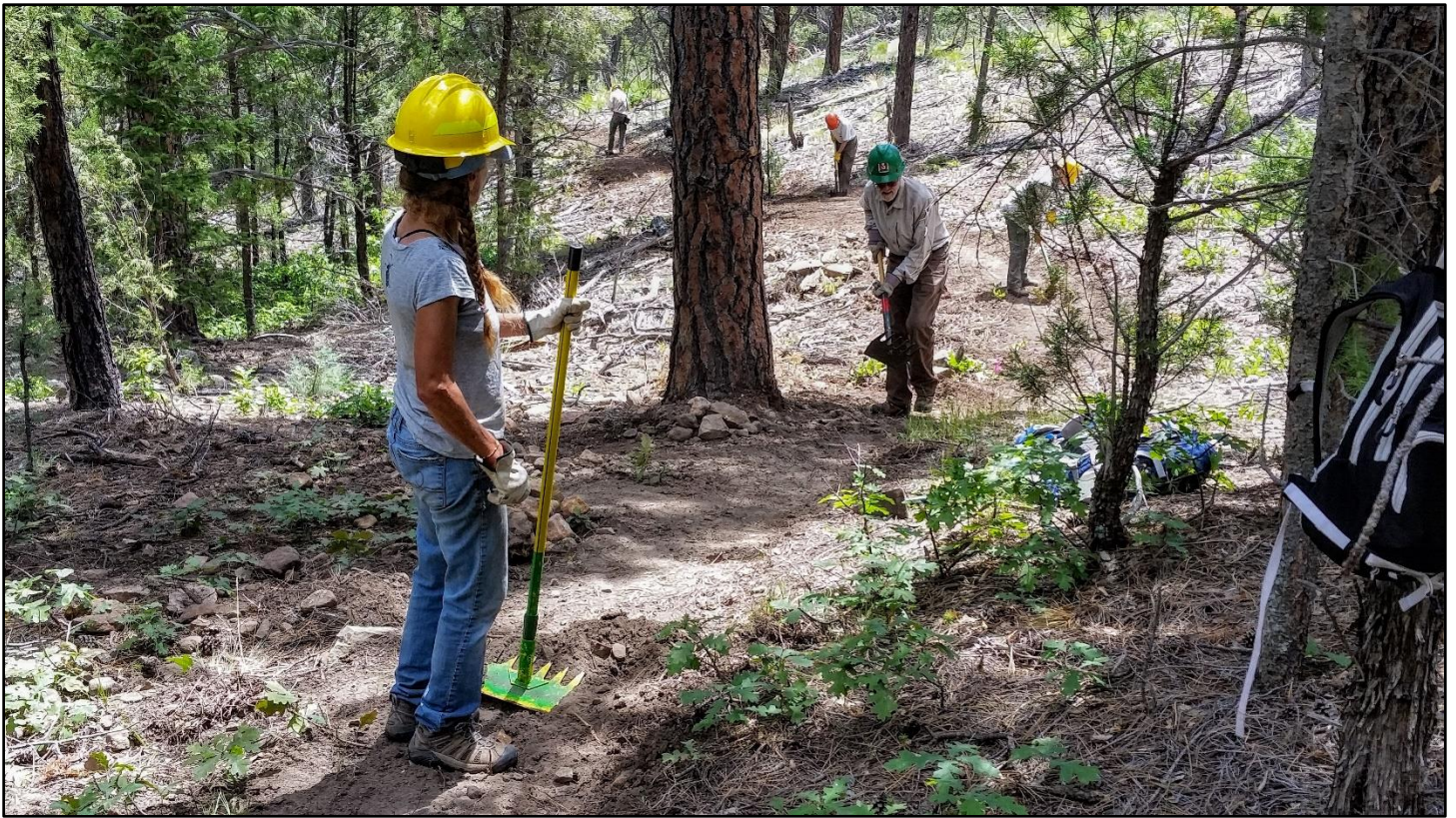
Tread and backslope cut last December are polished. Much colder then so we just hurried through it.
