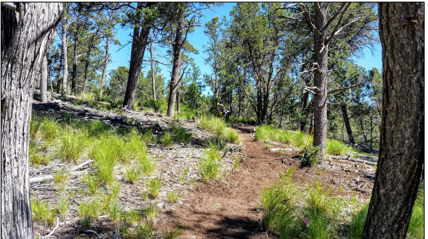
Nice finished tread down the slope. Working with an experienced crew is always good.
