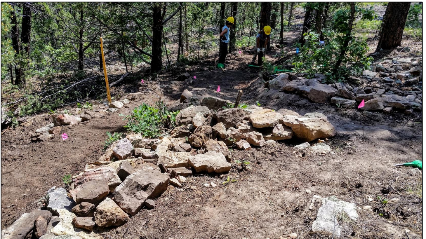
The upper connection is complete. The tread was basically cut in here by removing rocks.
