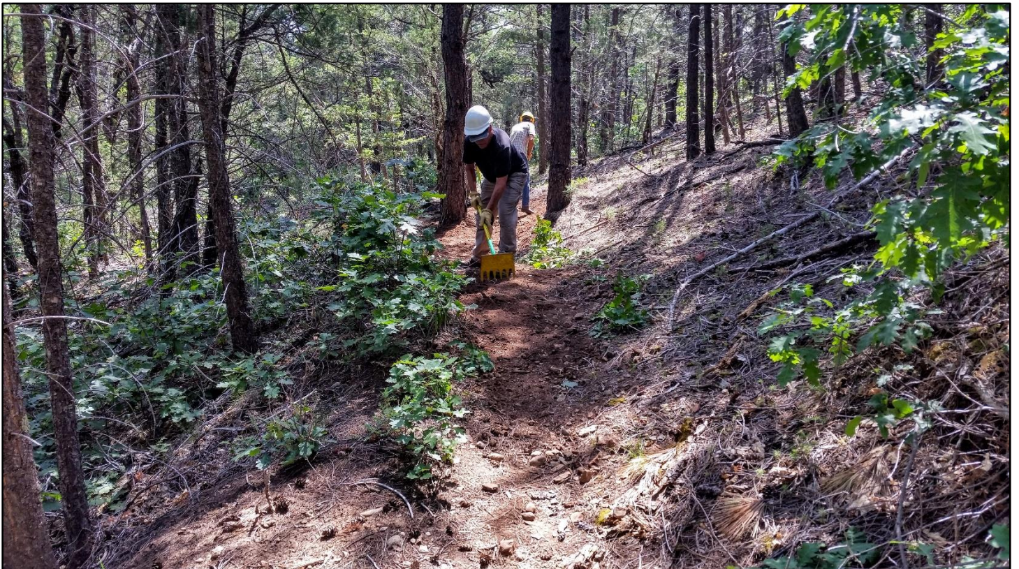
A smooth transition from the new trail section connects to the user trail.
