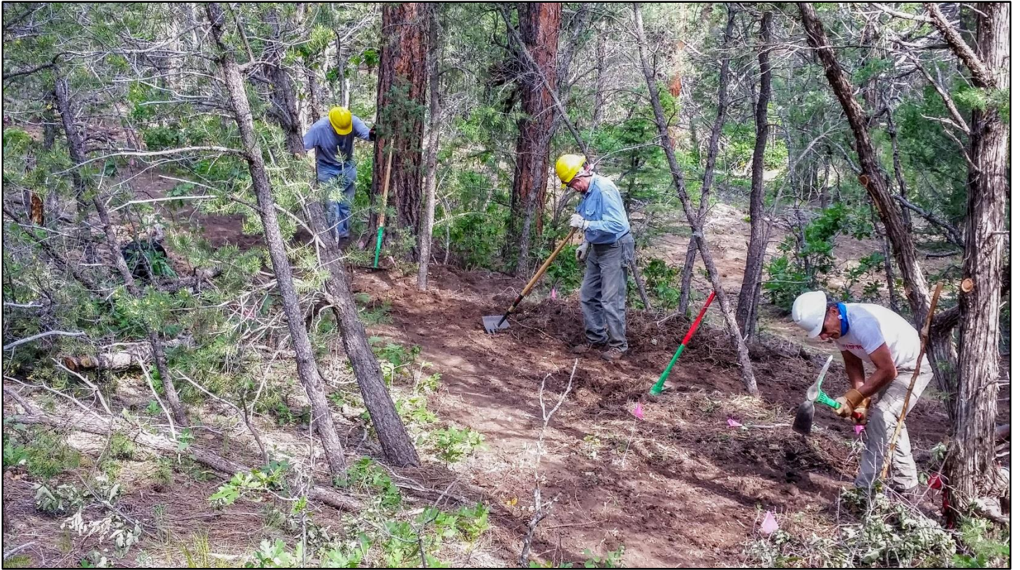
An intersection to the lower end of TC08 is cut into the trail headed up Cold Valley.
