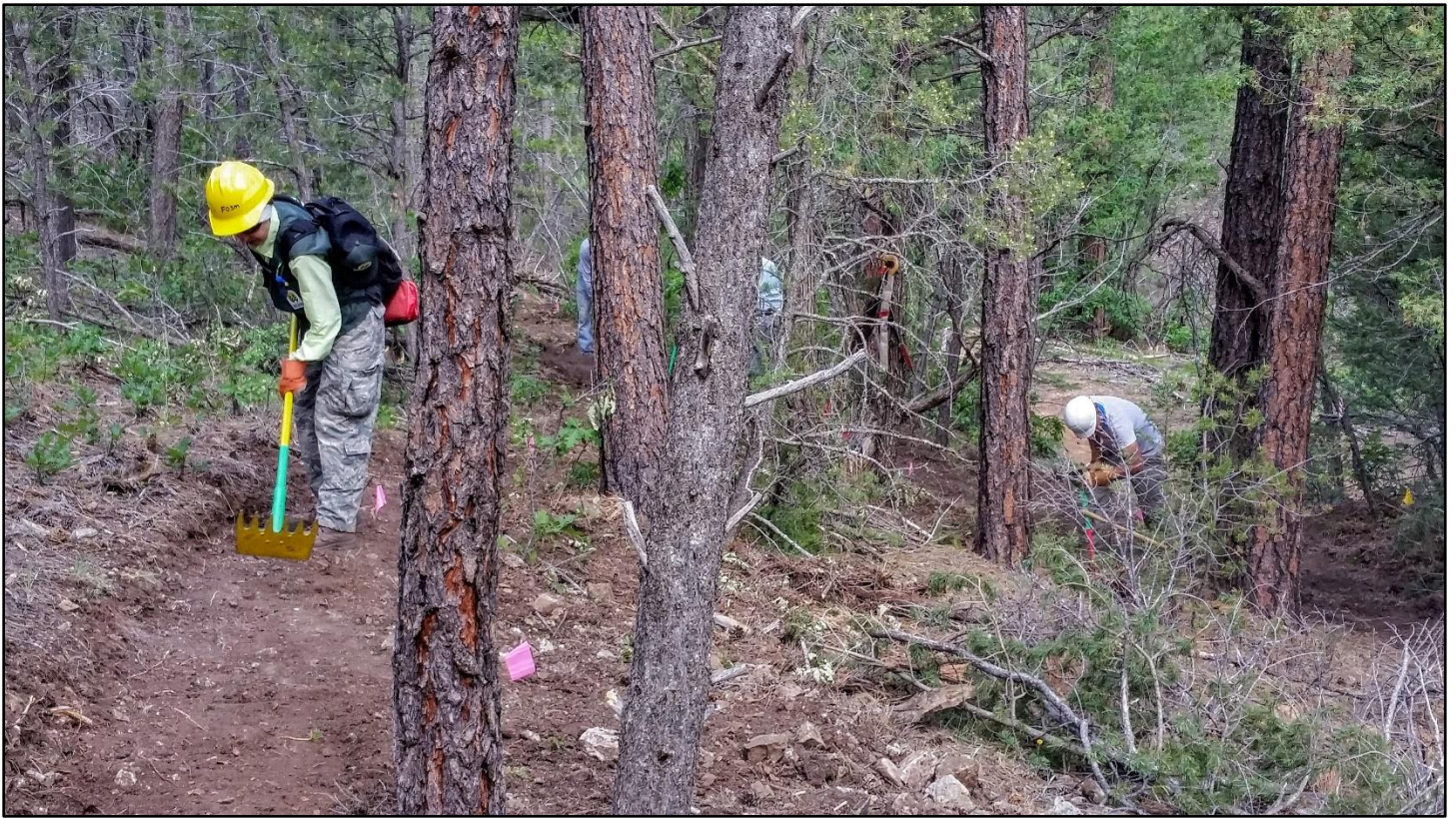
Final trail tuning down to the intersection. The bypassed section of old logging road was obliterated.
