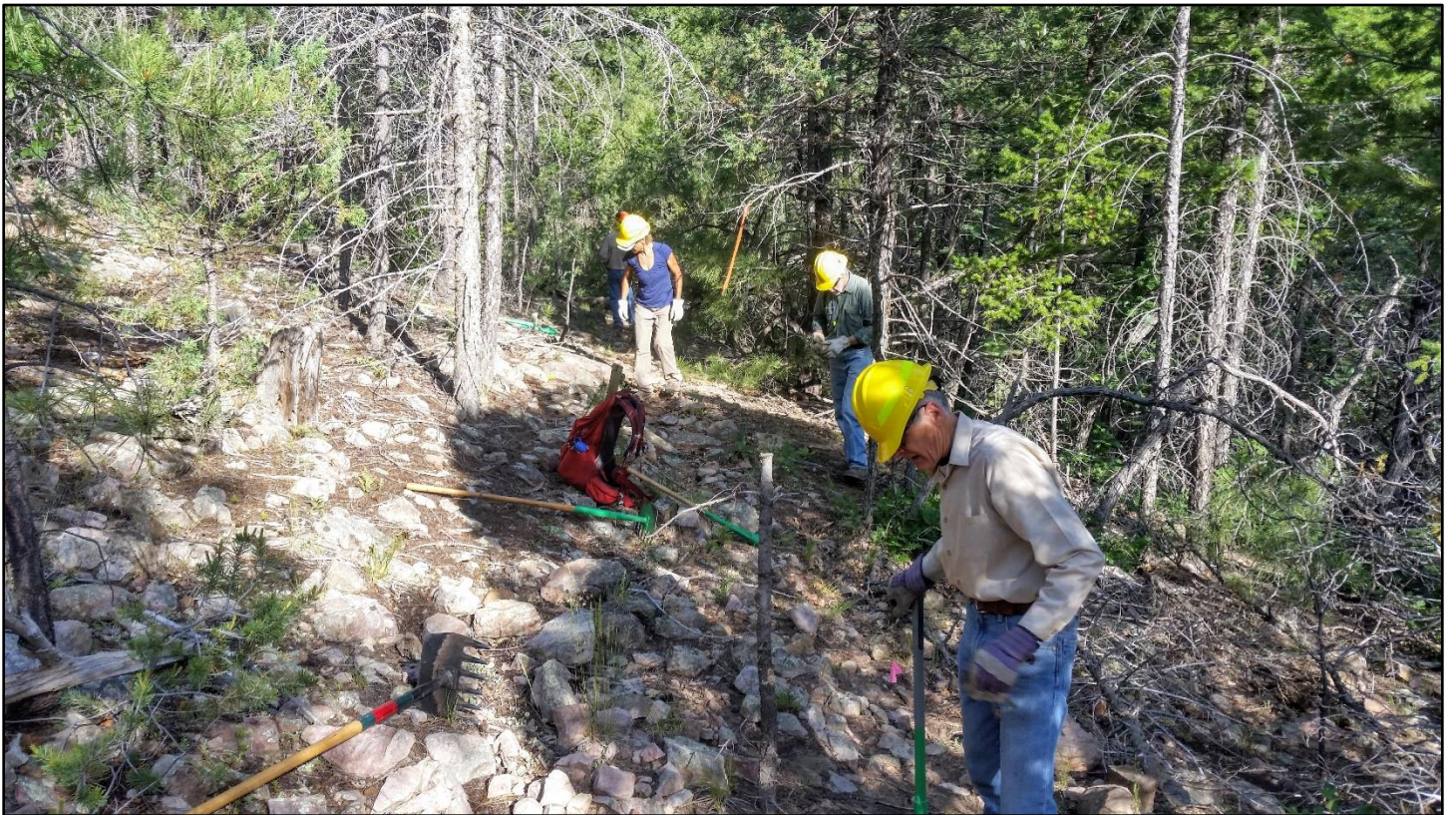
Before: Who boy! A lot of rocks to work through in this section.
