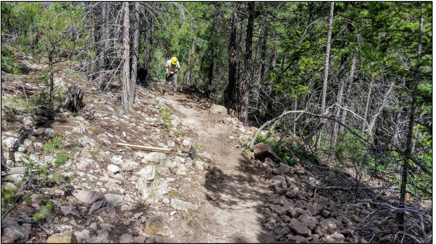
After: With many rocks removed, nice level tread was finally hacked out.
