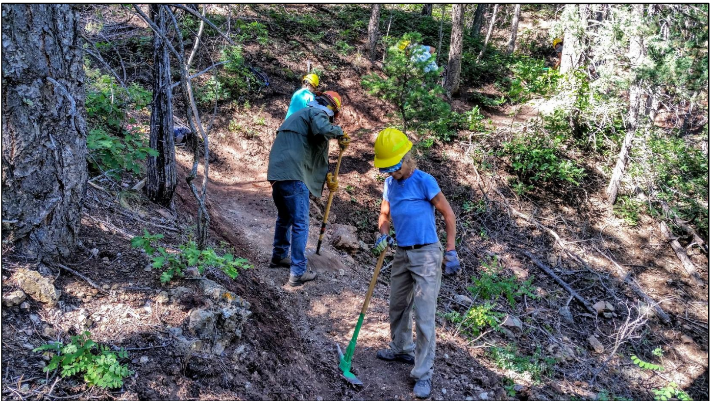
Much of this turn involved pulling out rocks and cutting back the steep backslope.
