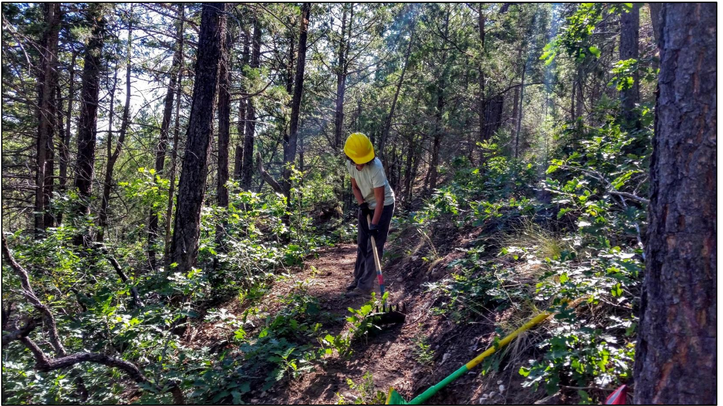
On the lower end of the section, a lot of oak had to be cut out and the tread leveled.
