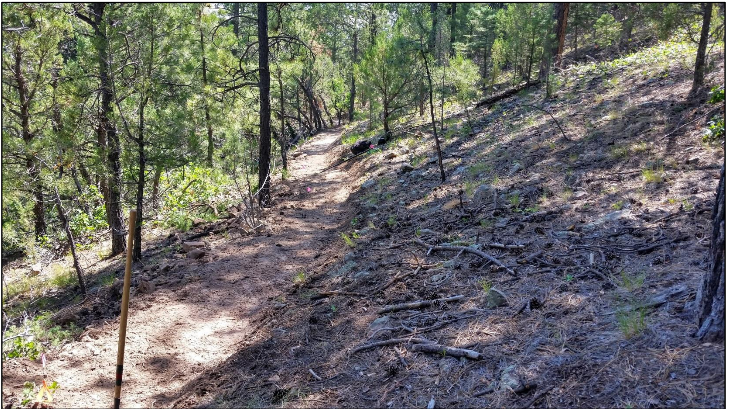
After: the sun burned through the overcast just as this section was completed.
