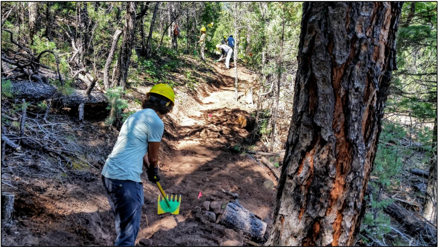
Final finish work on a new trail section. Some deadfall had to be cut off the trail here.
