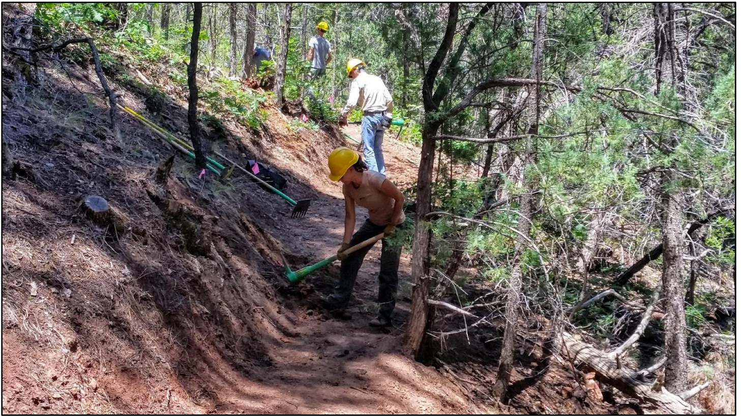
On the section completed earlier, the crew worked to cut back the very steep backslope.
