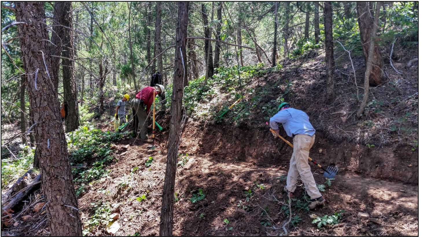
Quite a bit of effort was expended on the backslope and tread leveling.
