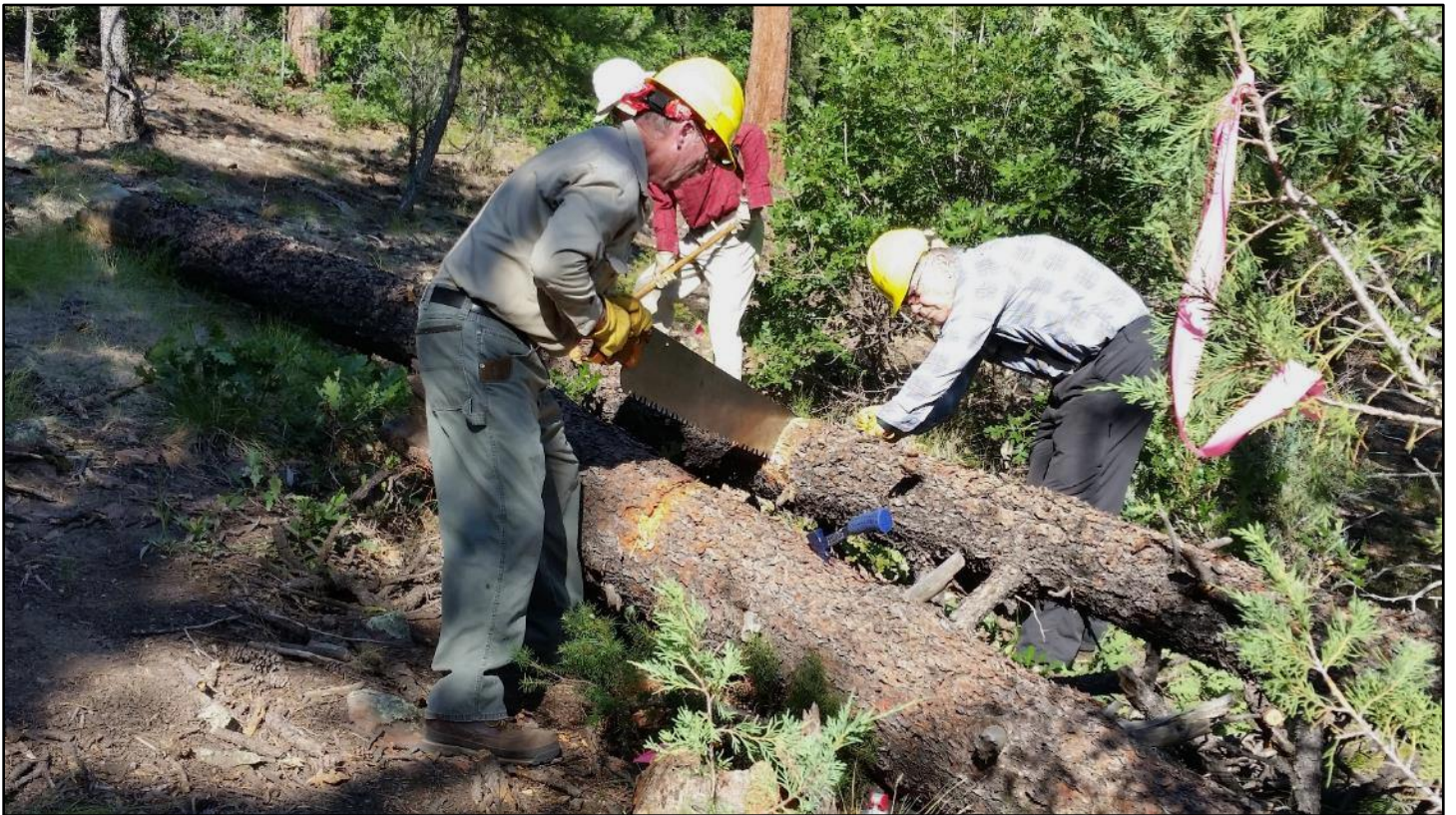
Meanwhile the crosscut sawyers started at the top of Section TC03 to open the trail corridor.
