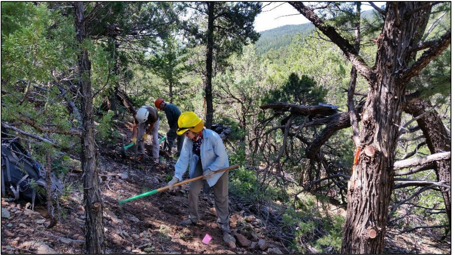
As the corridor opened up, the crew could start cutting tread. At least we were in the shade.
