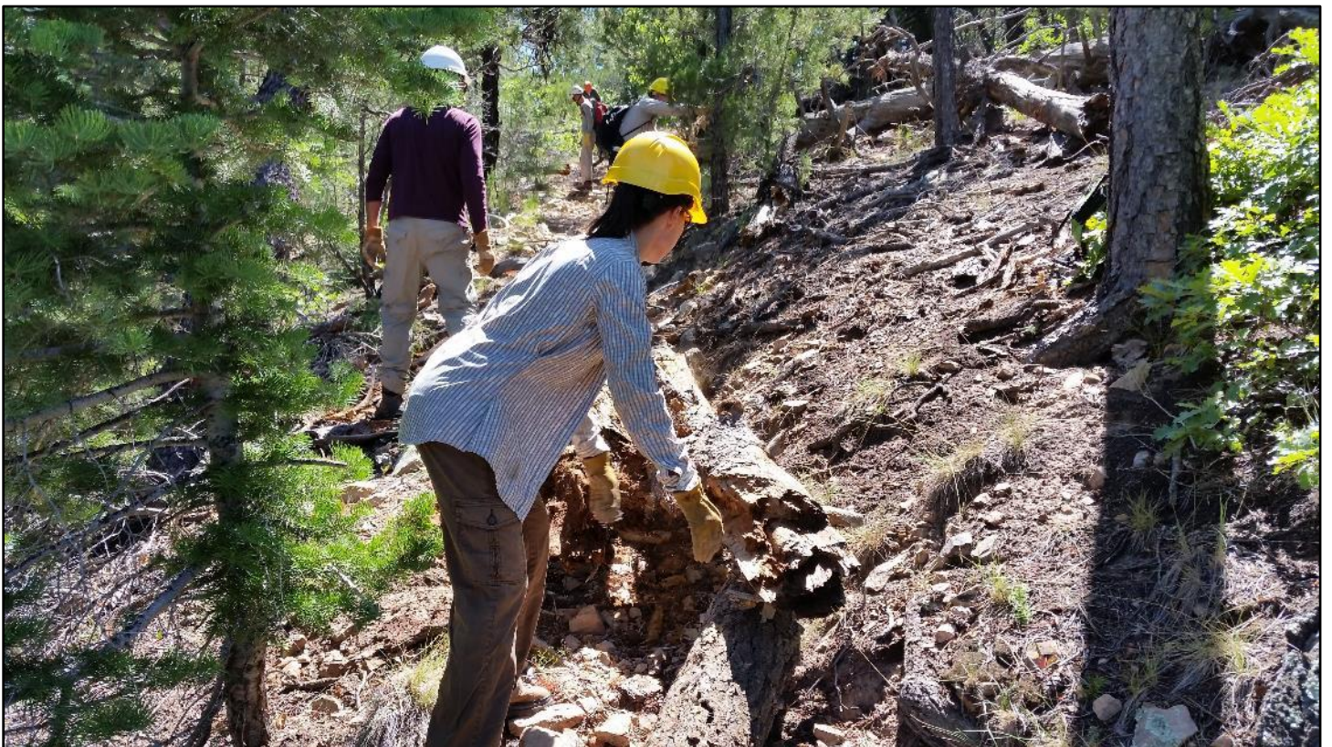
After lunch, obliteration began on the badly eroded user trail bypassed by the Madera Locura reroute.
