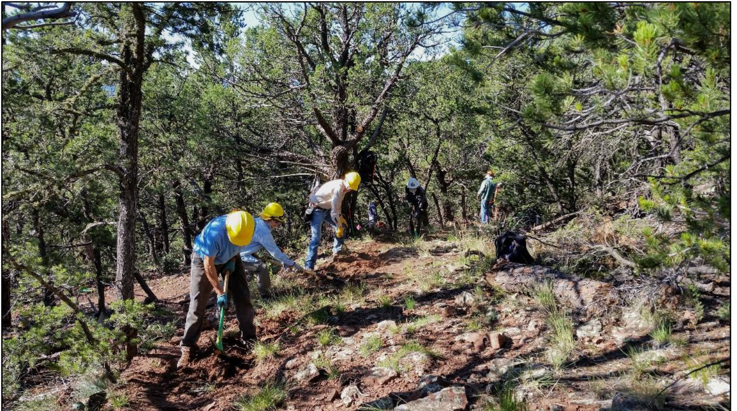
Part of the crew cuts in the upper end of a short reroute to bypass an eroding climbing turn.
