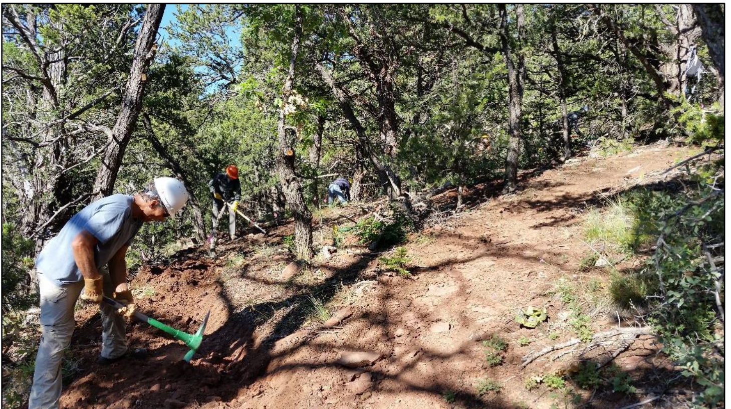
Before: Erosion in the steep turn on the right justified the reroute.
