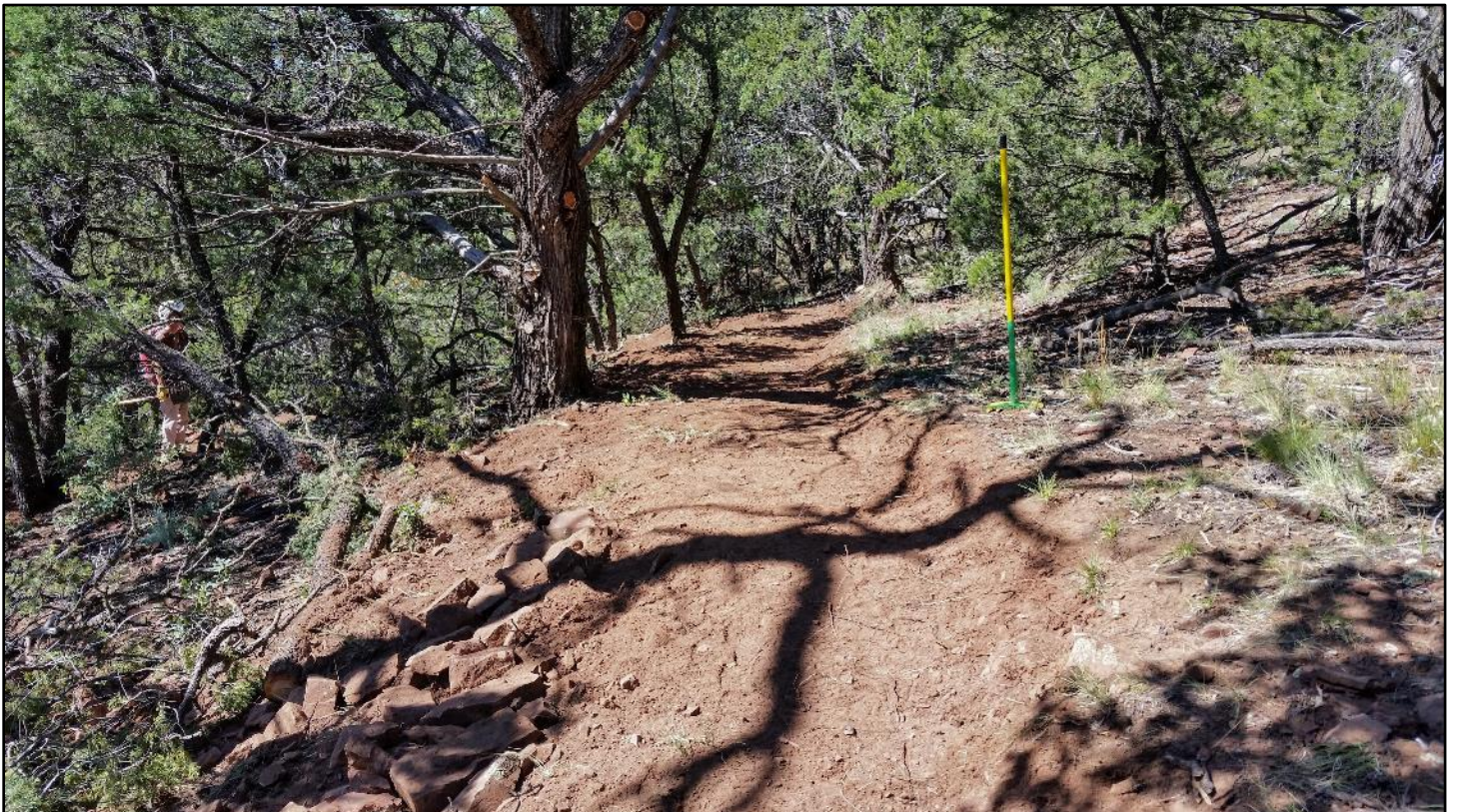
After: The upper end of the reroute is complete and the bypassed section obliterated.
