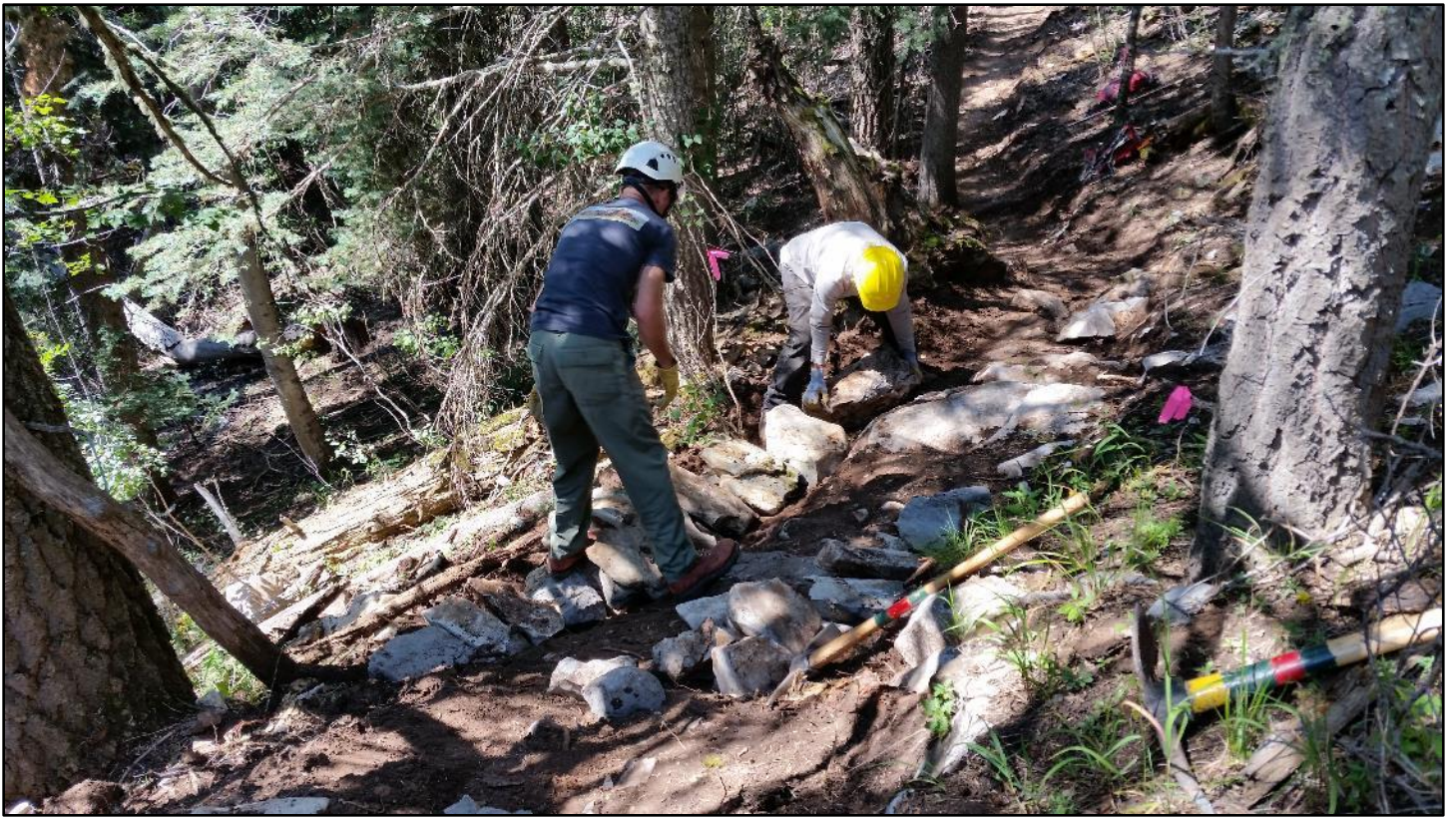
Cribbing work begins on a steep section studded with big limestone outcrops.
