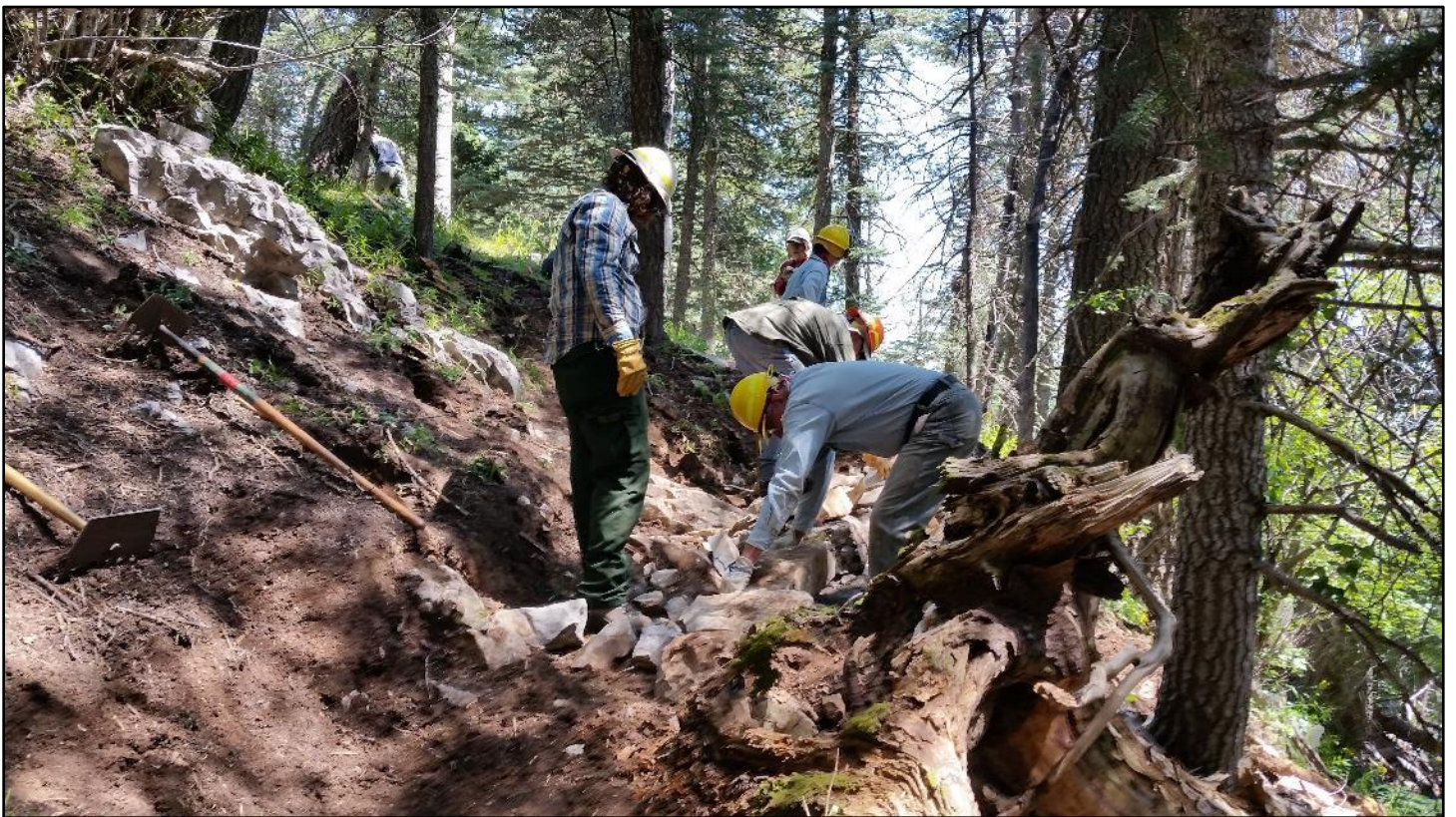
After lunch, additional horsepower was applied so the crew could complete the cribbed section.
