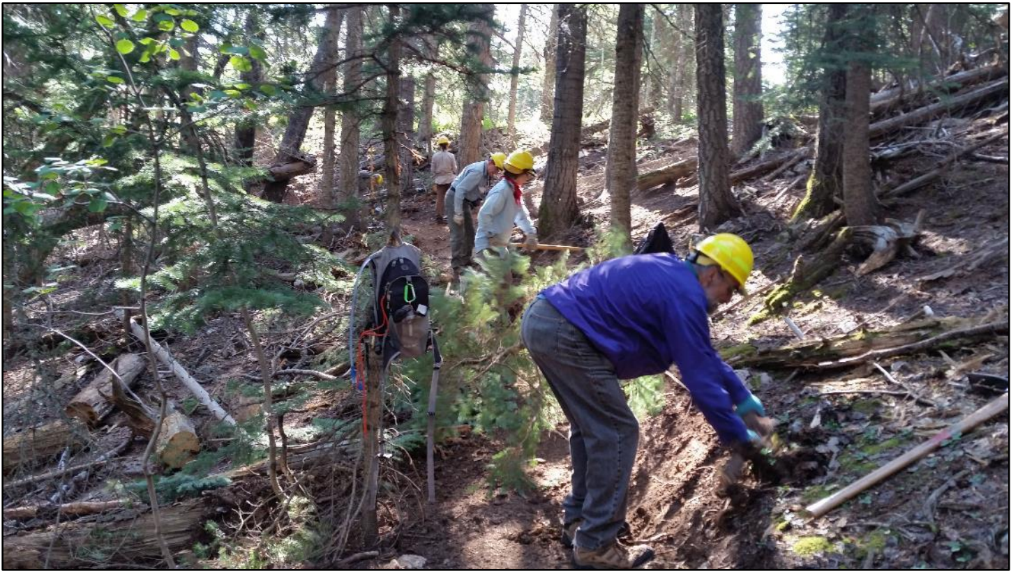
Much of the work involved sections of tread leveling, refining backslope, and removing forest debris.
