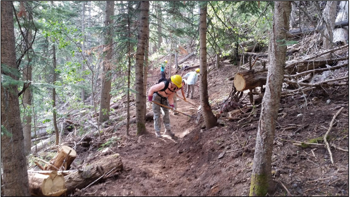
Grooming the backslope and clearing duff. Many compliments received from hikers passing through.
