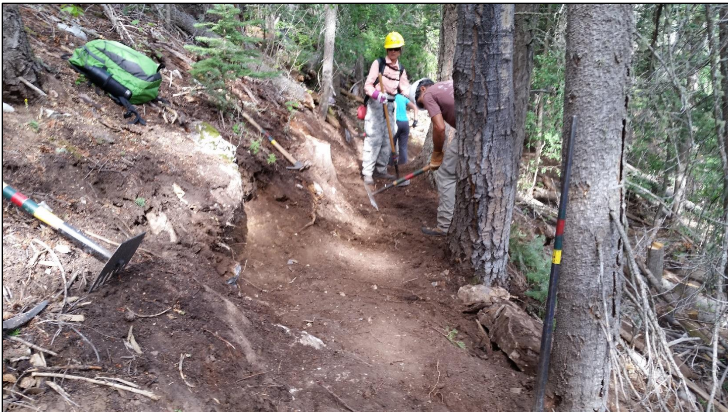
Done! The slab is pushed off to the the right and the trail finishers start to plow their way through.
