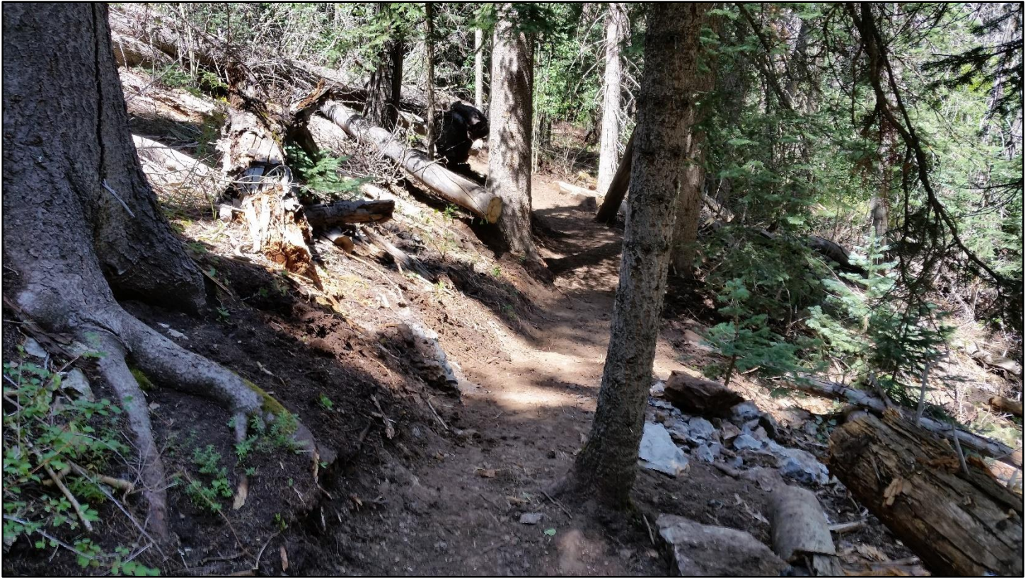
Boom, done! The narrow section is widened, producing a clear tread line.
