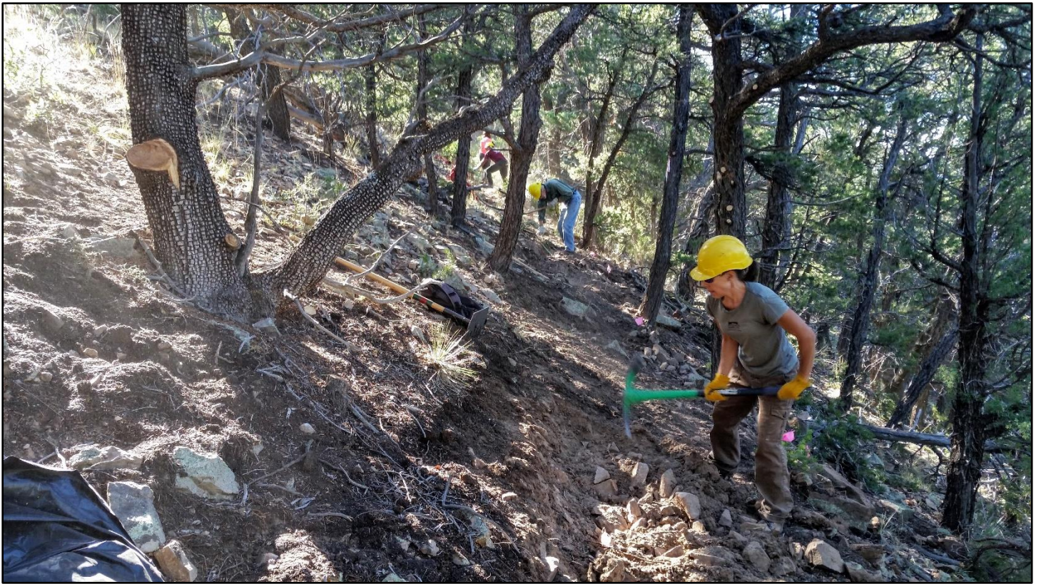
Steep slope and lots of rocks make for challenging tread cutting on Vista Trail.
