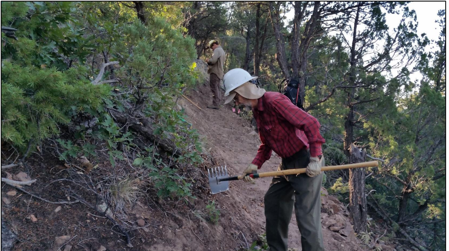
It is about a mile hike up to the work site; then the crew grabbed tools and pitched right in.
