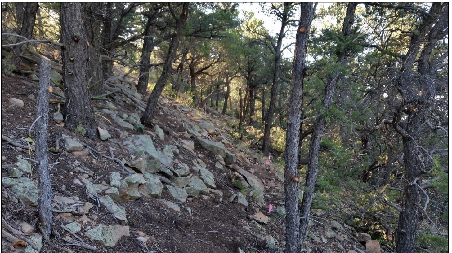
An example of the terrain the crew has to plow through to build Vista Trail.
