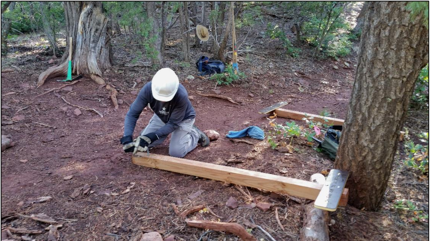
First step: install a deadman in each sign post. The crew started up at the Faulty Trail intersection.
