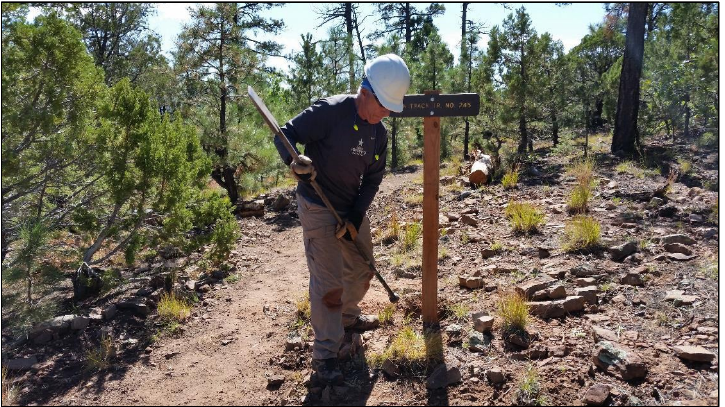
The hole for the Elk Track Trail sign hits 24 inches: level the sign and pack in the rocks.
