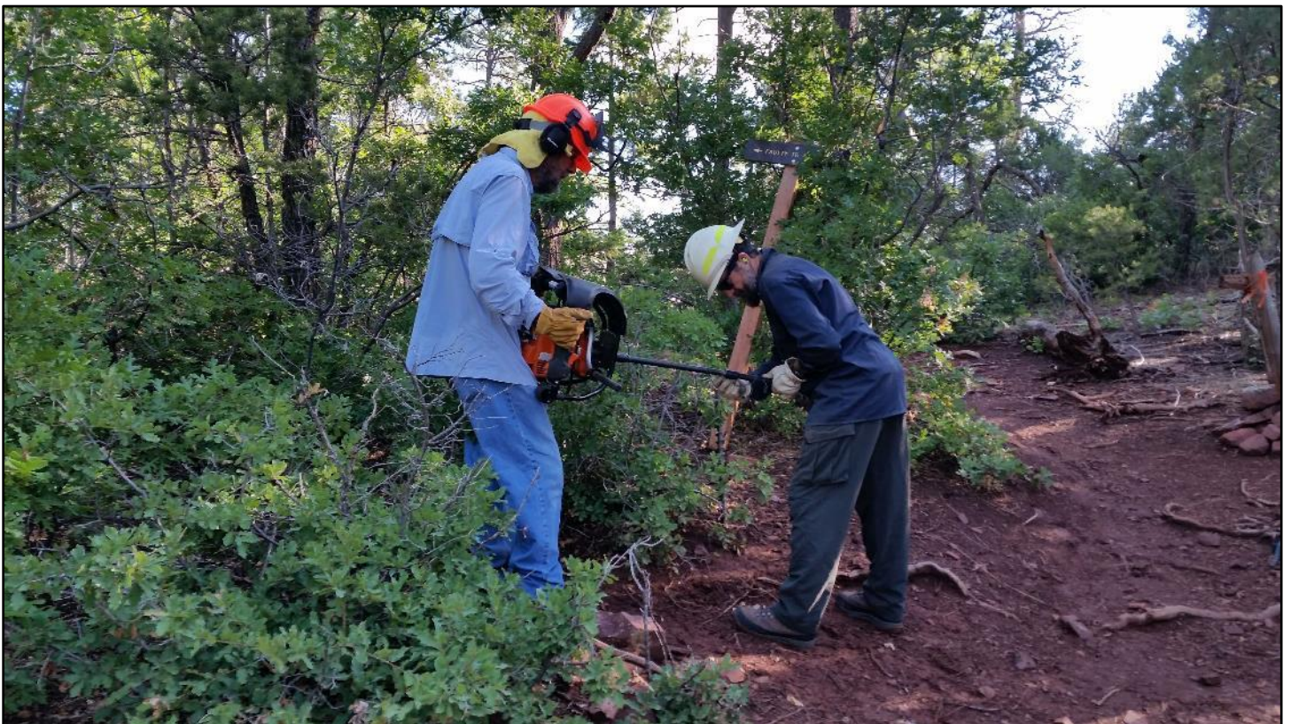
Bit change-out on the power auger. Hmmmm, this red caliche is REALLY compacted.
