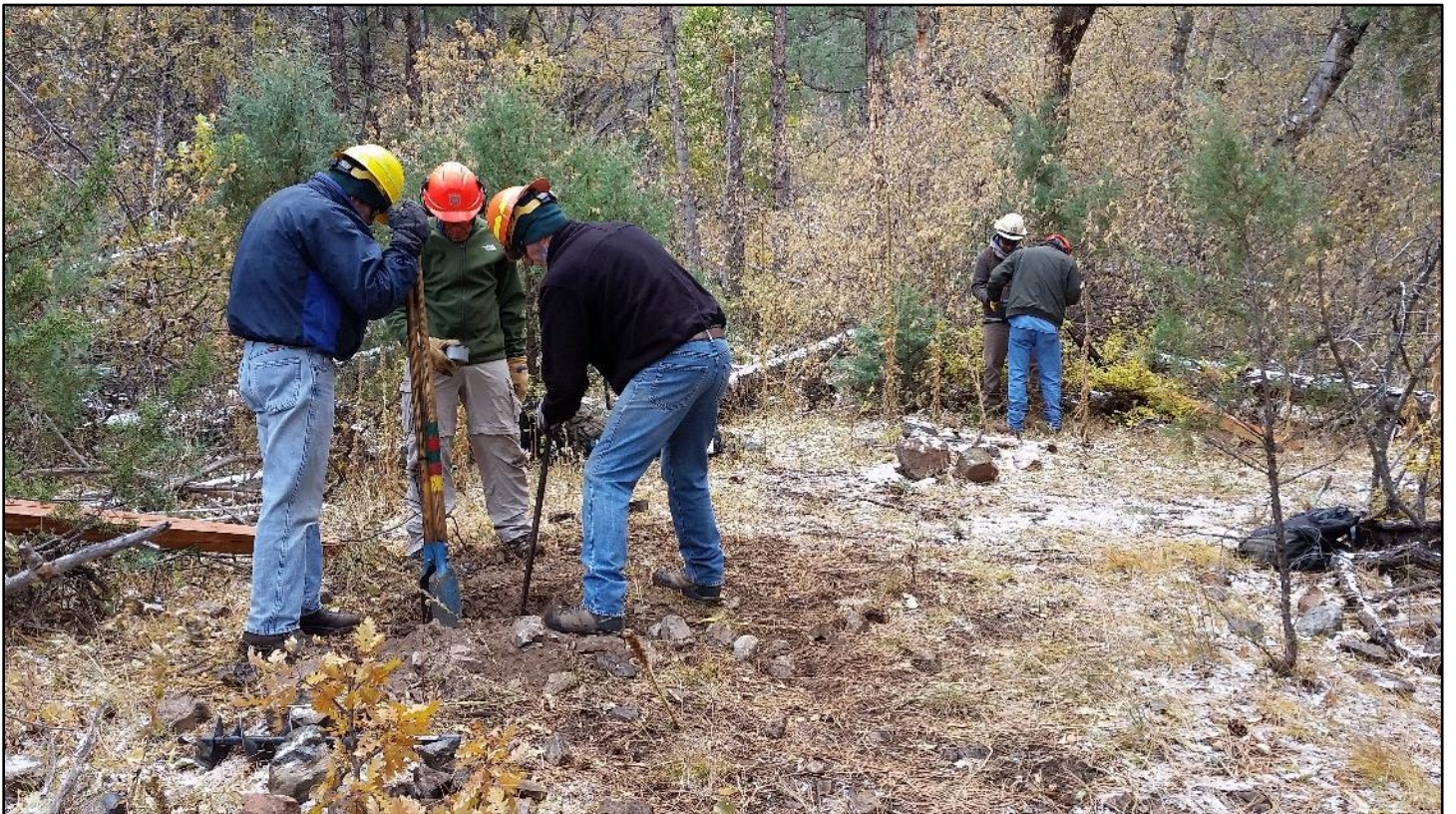
The first hole nears the required depth while the auger crew gets after the second hole.
