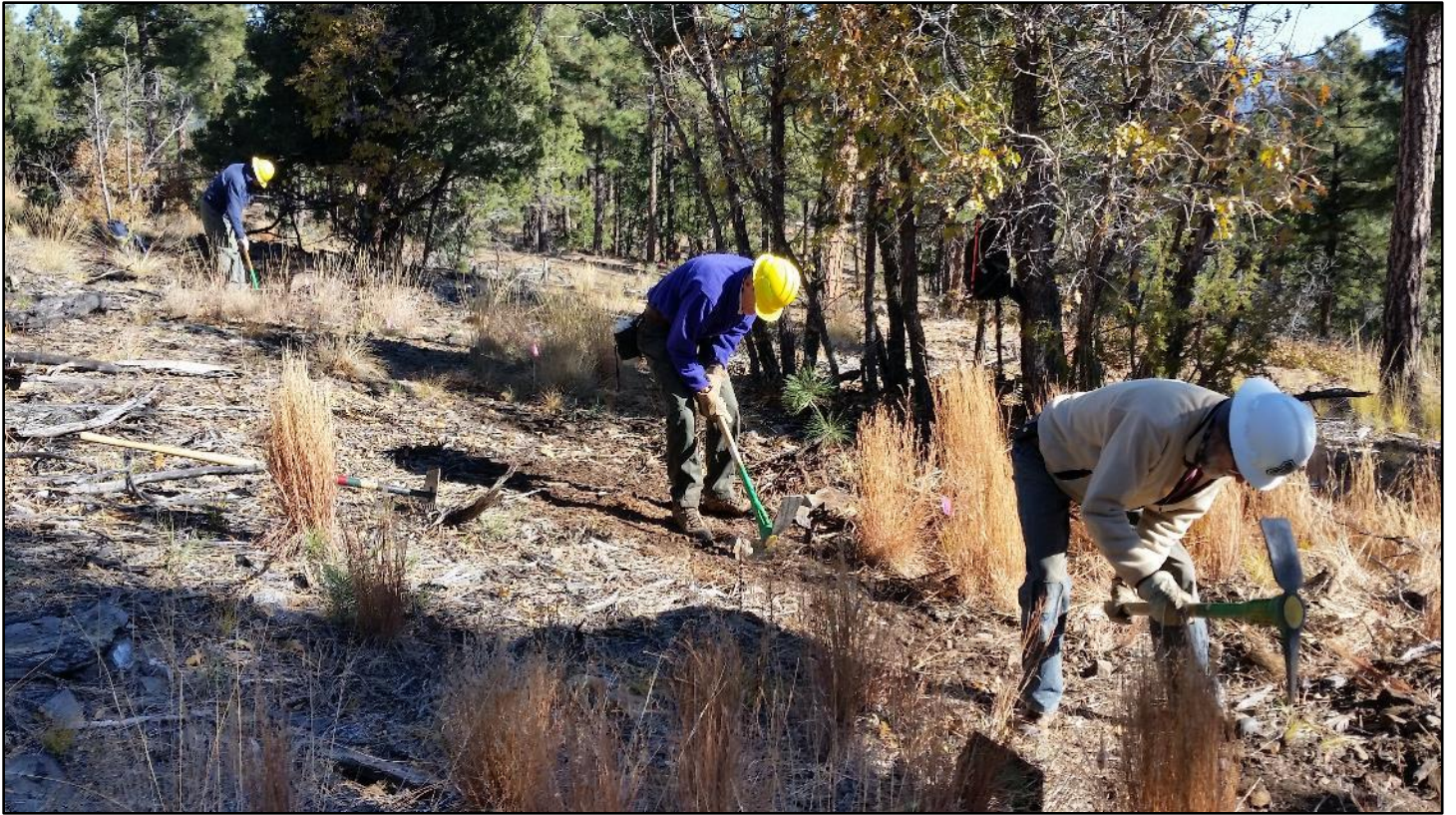
The FOSM pick operators line up to pull the many rocks and level the tread.
