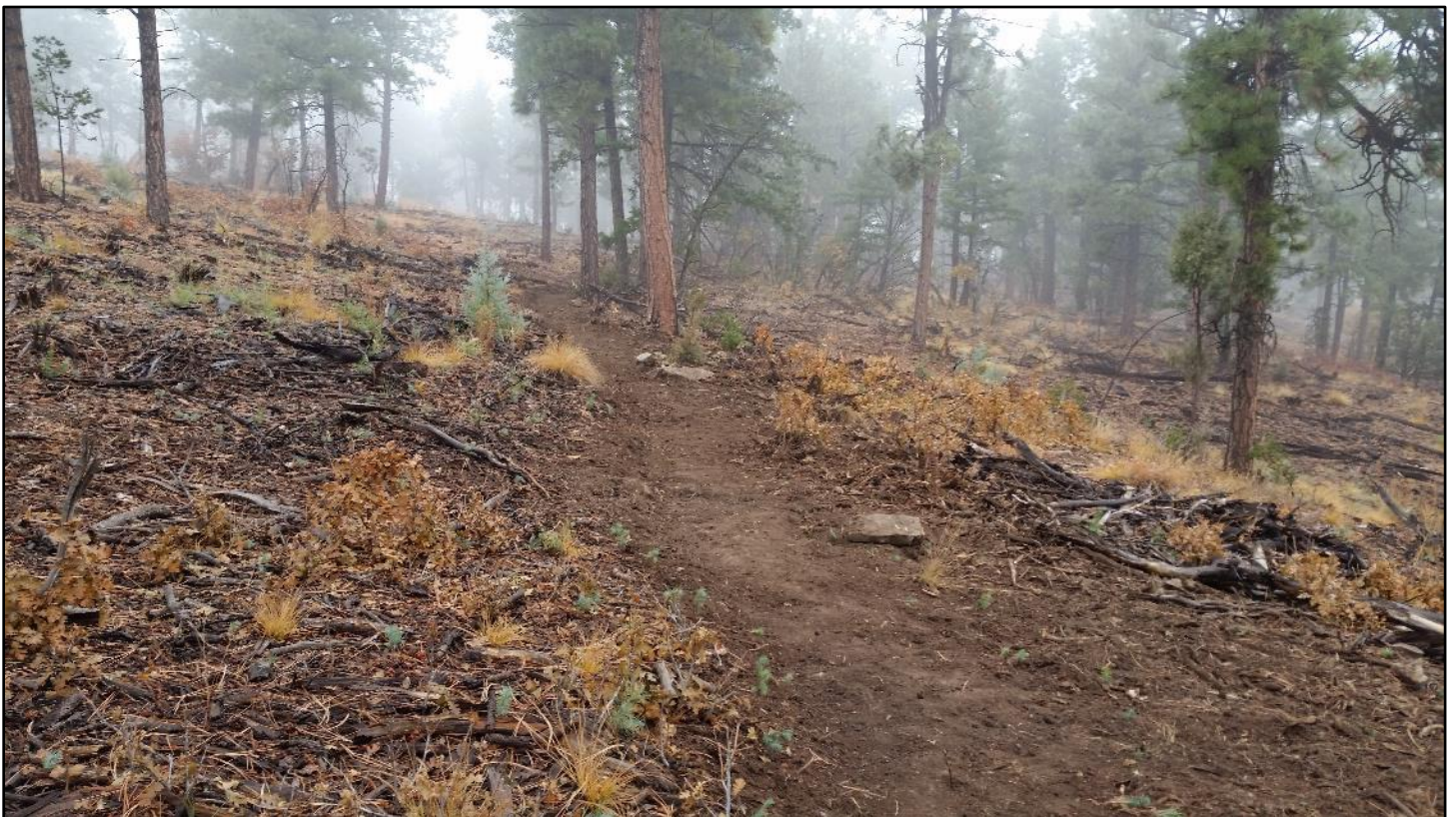
After: the result when the crew is finished is nice sustainable trail down the slope.
