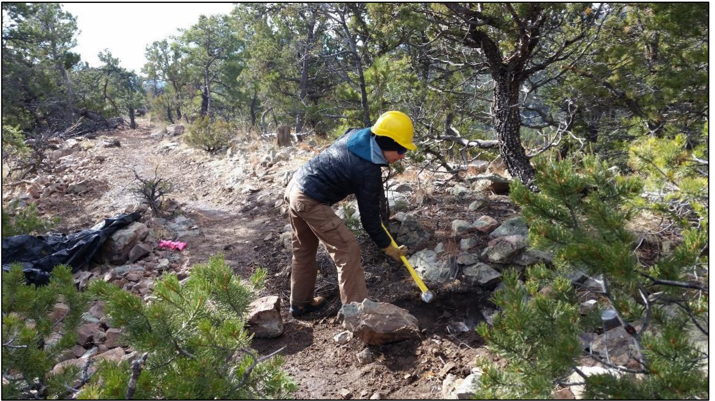
This hole was more of a challenge. The “persuader” was drafted for this rock outcrop.
