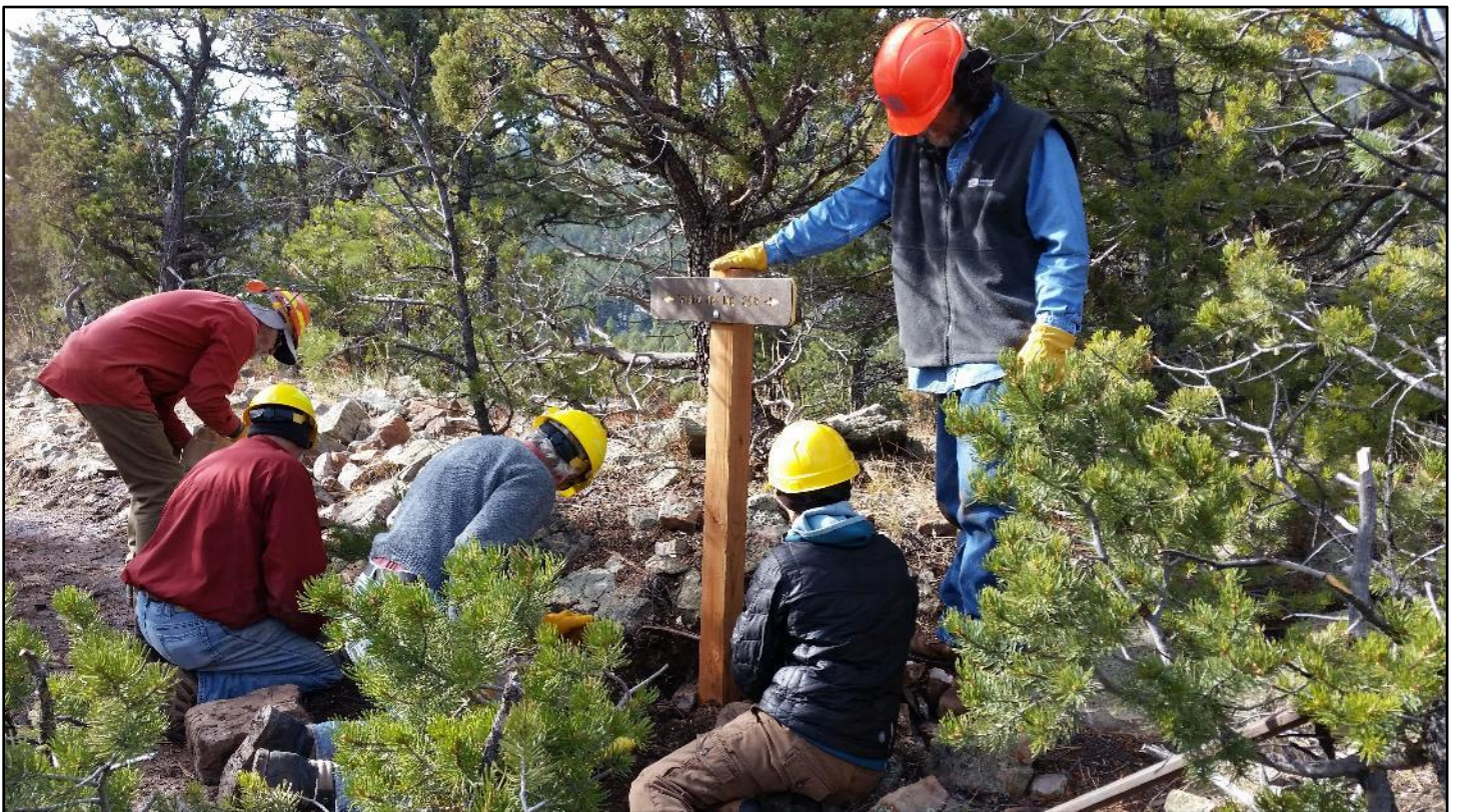
Ok, we had to get the whole crew packing this one into the cleft in the rock outcrop.
