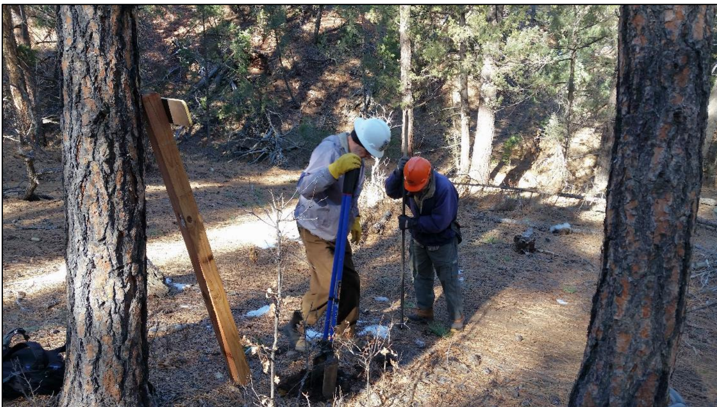
No auger was needed. The moist soil had few rocks, requiring minimal coaxing from the digging bar.
