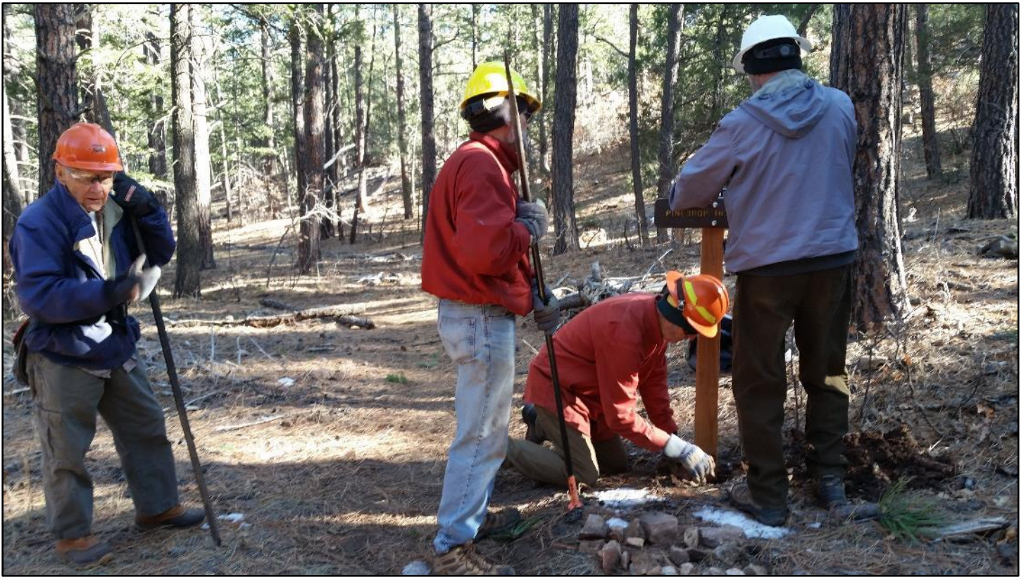
Packing in the rock fill. Many rocks were frozen to the ground and had to be pried out.
