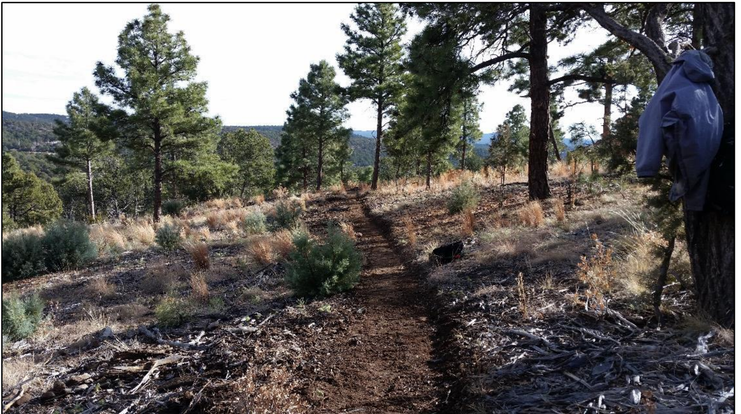
In spite of the challenging conditions, the small crew still managed to cut 425 feet of nice new trail.
