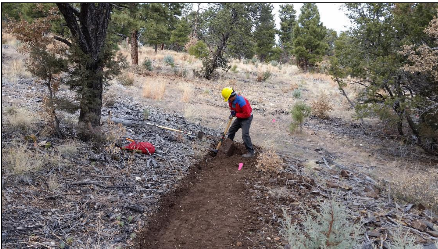
Some sections actually had more dirt than rocks. Ok, this guy did manage to find a boulder...
