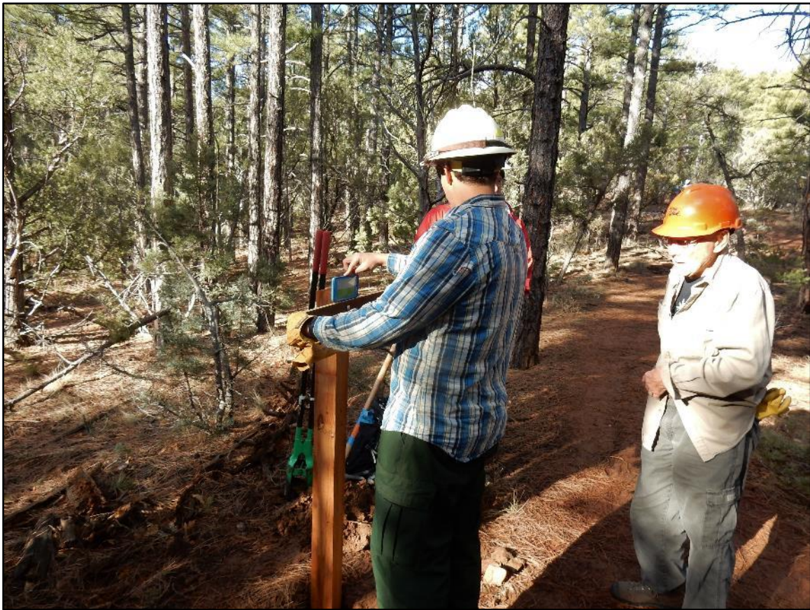
Making sure the Cresta Trail sign is level. Over-engineering is never a bad thing.
