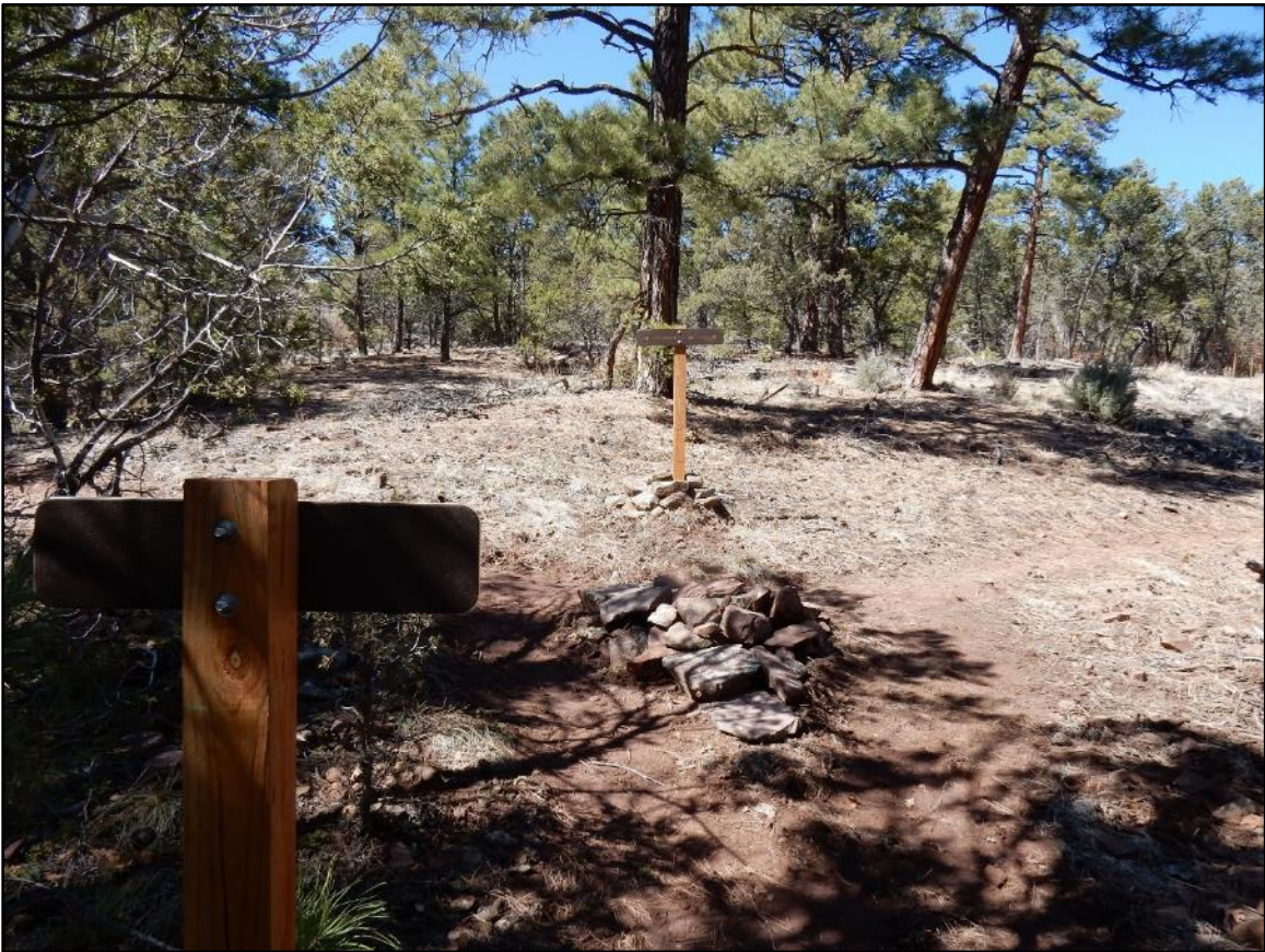
Finally finished! We ran into plenty of rocks here but both signs are in.
